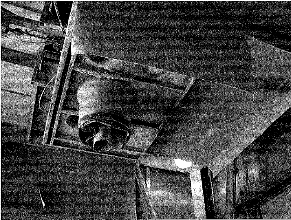
Image 1(Photo 1) : Hood with two intake points to collect dust from truck loadout.
