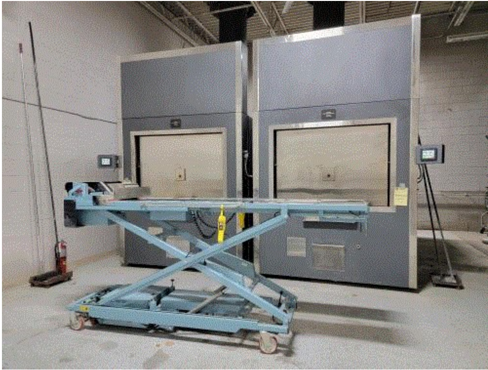
Image 3(20221215_094221) : EUCREMATORY6 (left) and EUCREMATORY5 (right), with a lift table in front. The lift table has a ram that is used as a mechanical assist when inserting a charge. The operator attaches the table to the cremation unit to maximize control.
