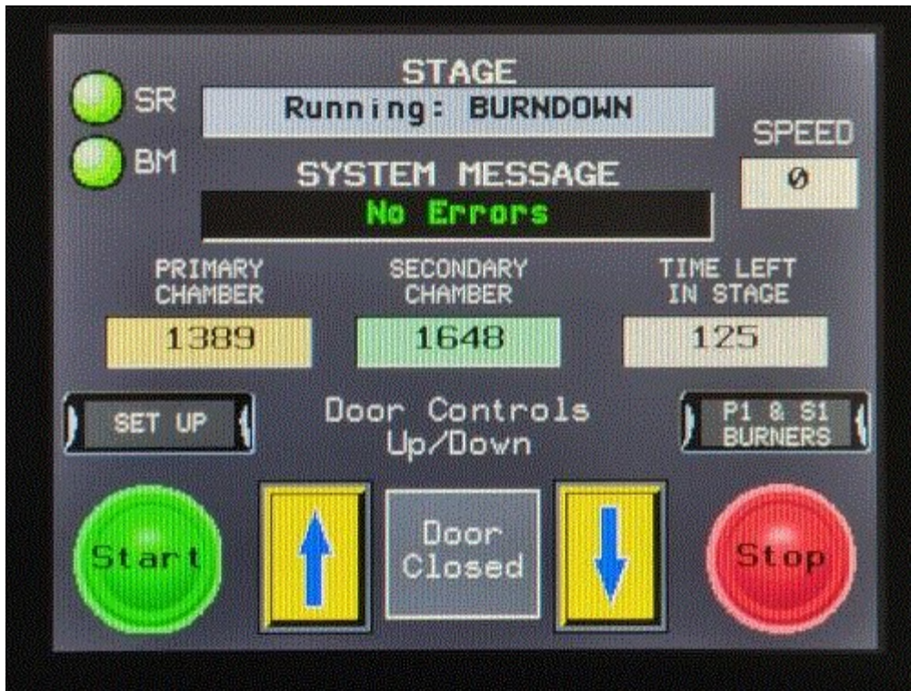
Image 4(20221215 094259) : Close-up view of EUCREMATORY5 digital control panel.
