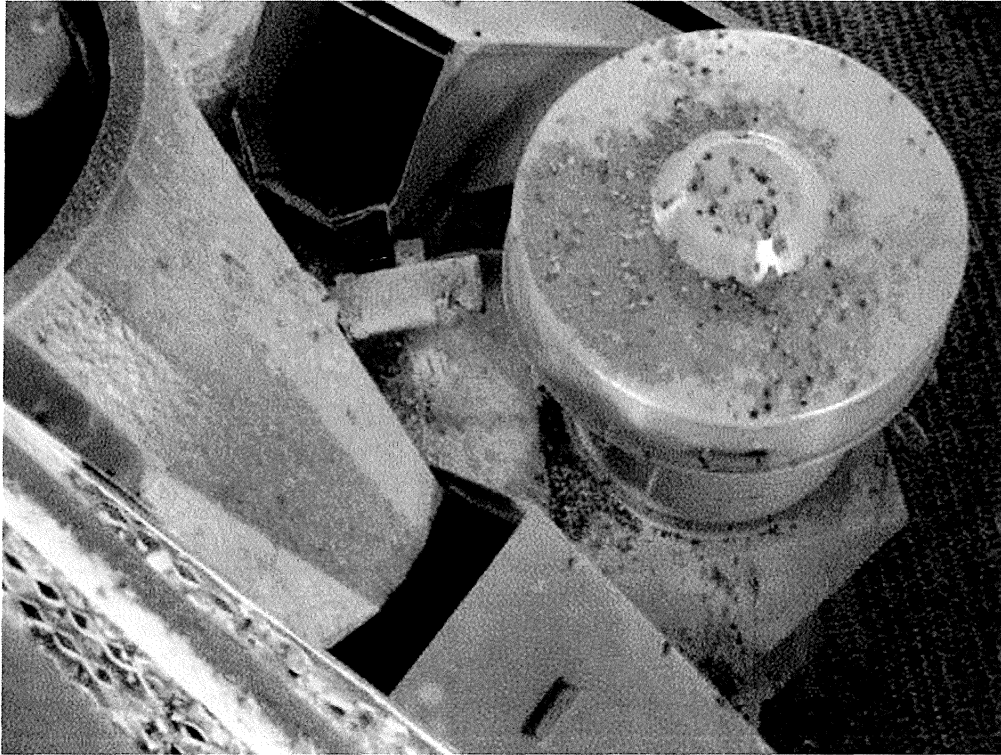
Image 3(003) : New baghouse, for silo control.
