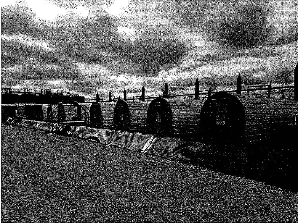
Image 2(Heater Treaters) : Heater Treater oil/gas separation units
