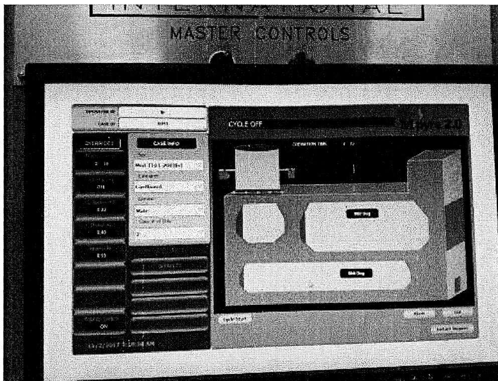
Image 10(Control Panel) : Control Panel-new incinerator.
