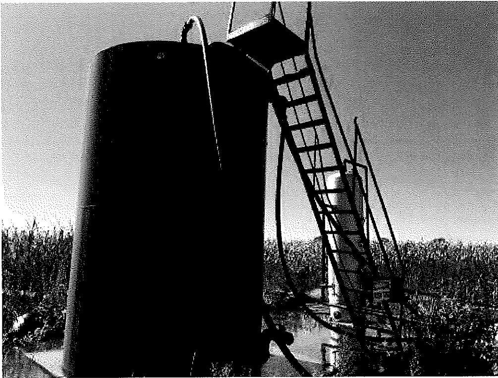
Image 1(Photo 1.) : Photo 1. Reference photo of storage tank and separator.
