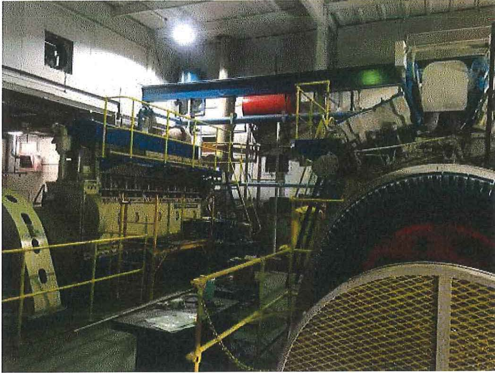
Image 3(Units #3 and #4) : Worthington generators
