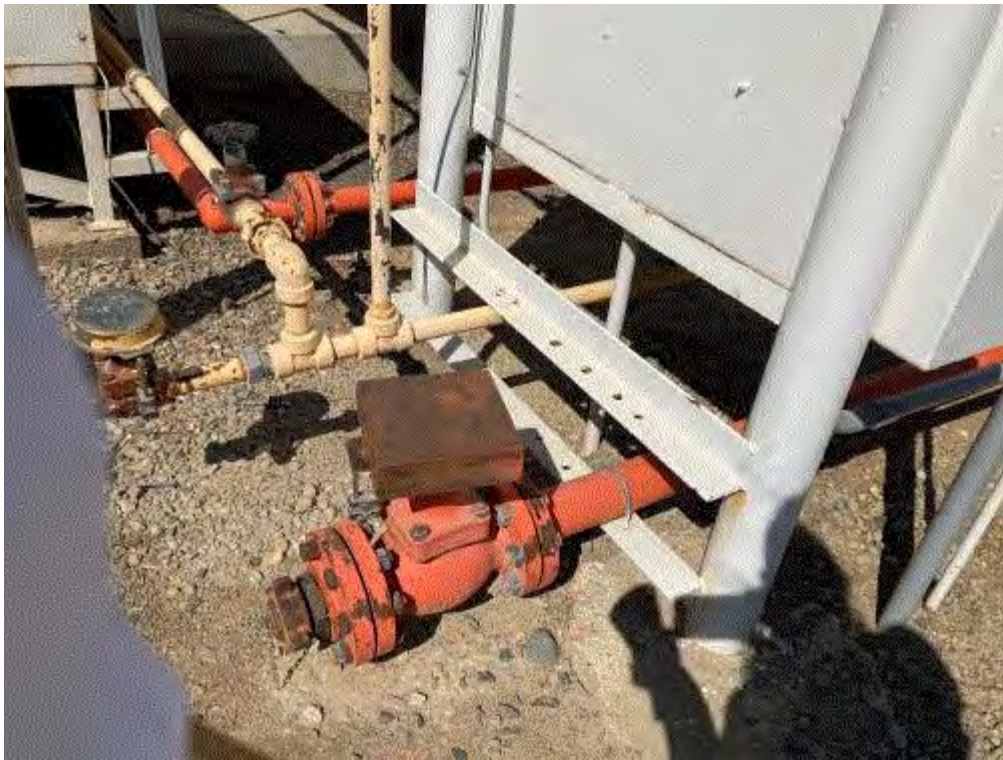
Image 1(Vapor & Liquid Lines) : Vapor and liquid lines without labels during inspection.
