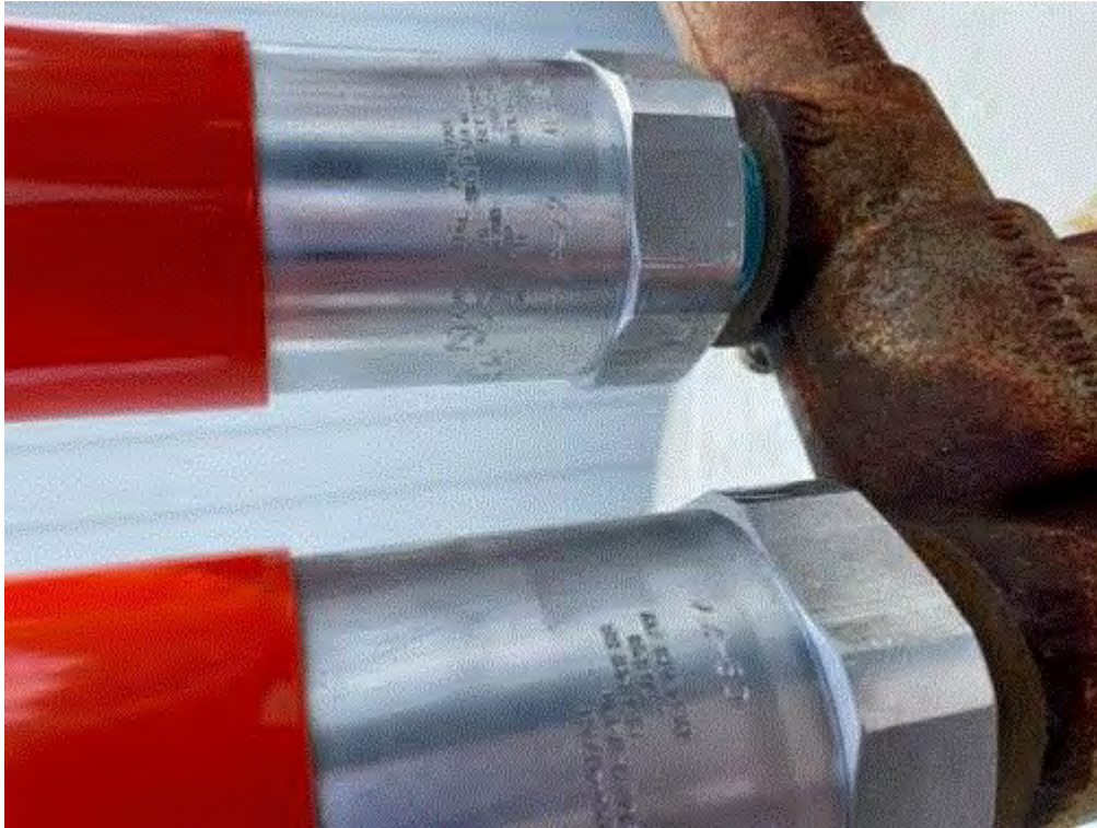
Image 3(Safety Relieve Valve) : New Safety Relief (Pop-off) valves installed post-inspection. (Photo courtesy of Scott Turner).
