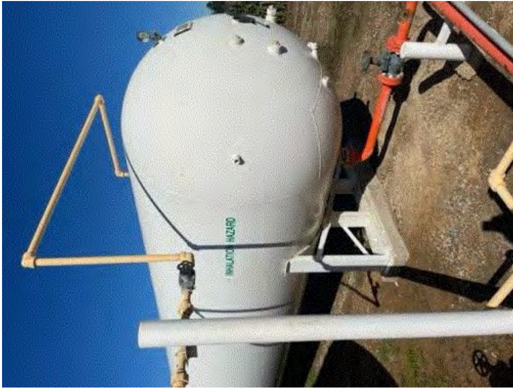
Image 5(Tank Labels) : "Inhalation Hazard" labels added to call tanks to ensure present on both sides of tank. (Photo courtesy of Scott Turner).
