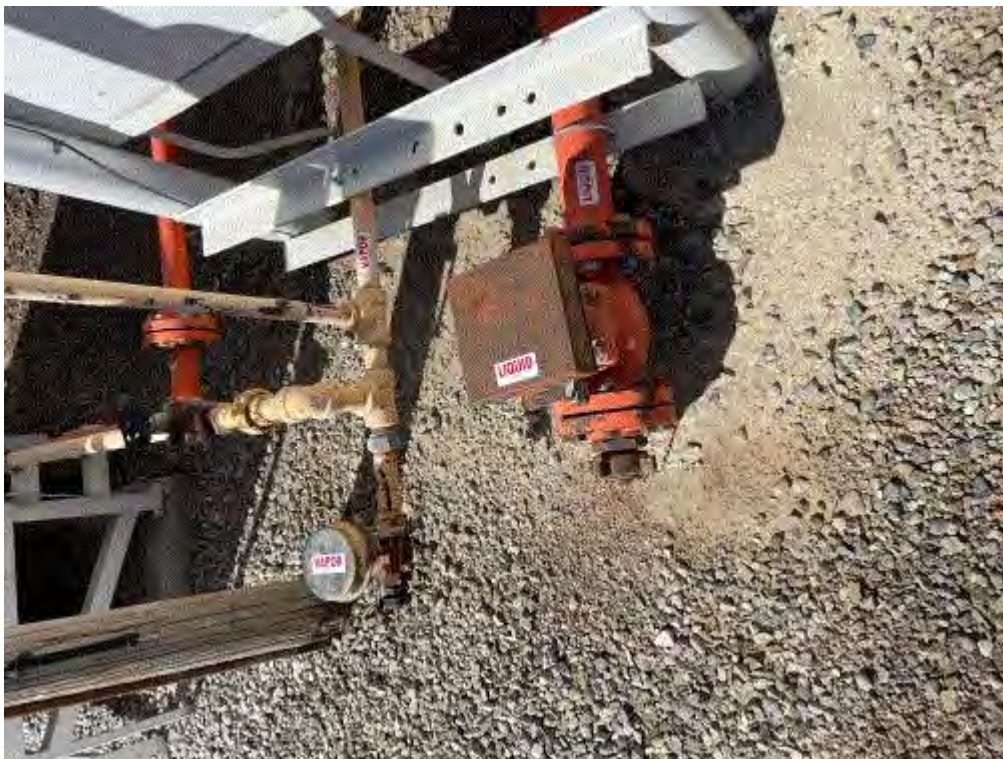
Image 2(V & L Lines - Labels) : Vapor and Liquid lines labeled appropriately (photo courtesy of Scott Turner).
