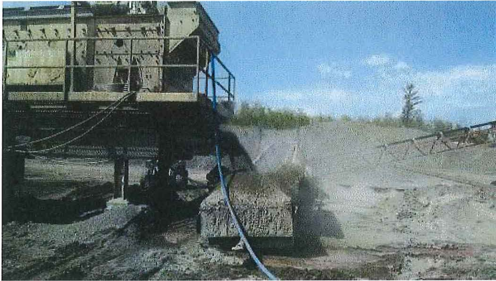
Image 3(Crusher w/ new spray) : Crusher 85102 with new spray bar installed. June 1, 2017
