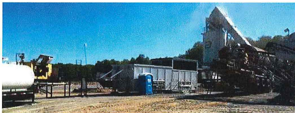
Image 3(C343) : Water tanker, control room, silo, drum
