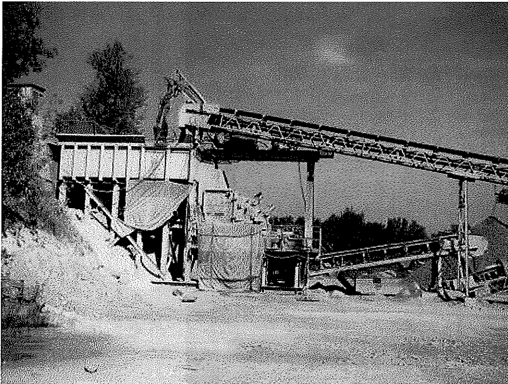
Image 3(Conveyor System) : Feeder Hopper, Primary impactor, and Conveyors 1 and 2
