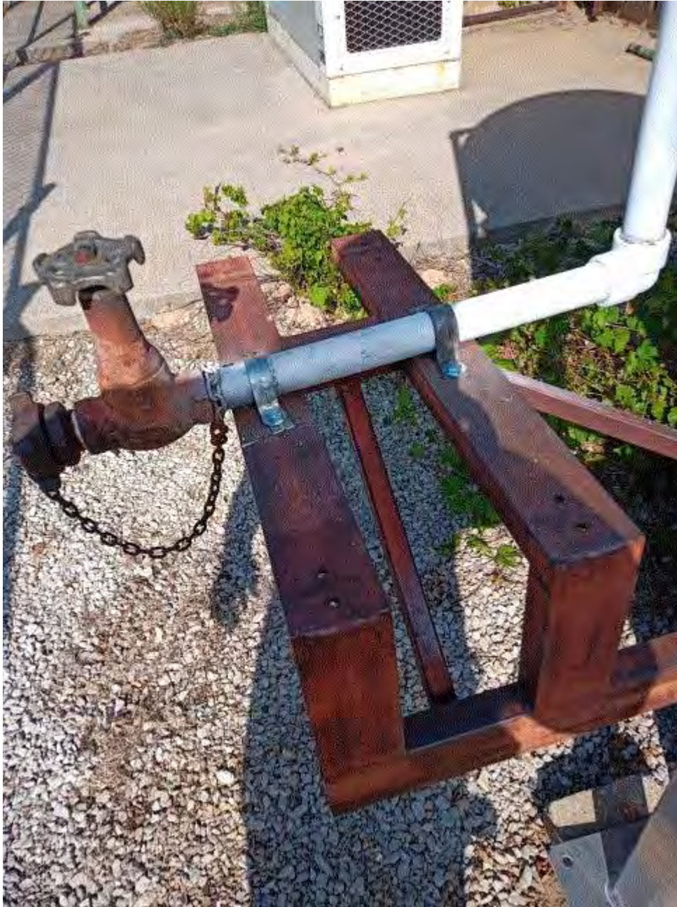
Image 3(Supported transfer) : Support transfer lines. Note Nitrex installed bolted "straps" to ensure the transfer lines were secured to the support structure to ensure a predictable breakpoint.
