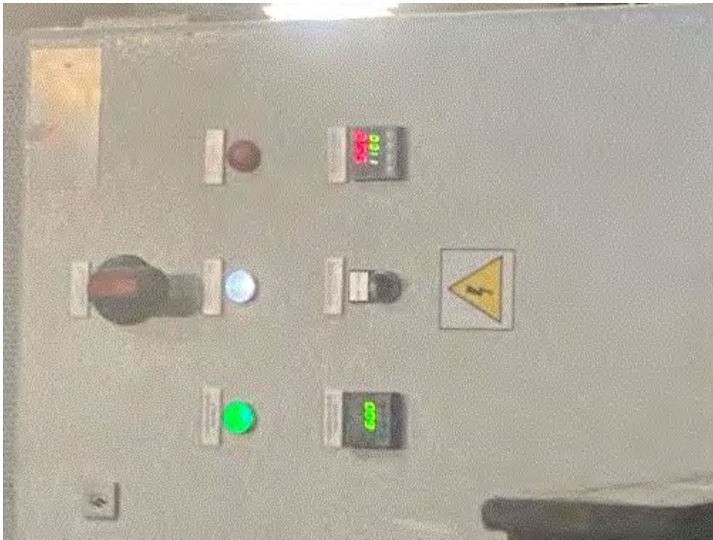
Image 4(N37) : N37 Neutralizer control panel with monitors for the burner temperature and the overtemp temperature.
