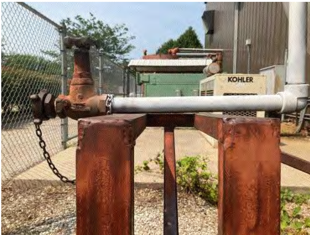
Image 2(Bulkhead) : Bulk head for anhydrous ammonia transfer lines. Note gap between pipe and metal support structure (not secured to support structure).
