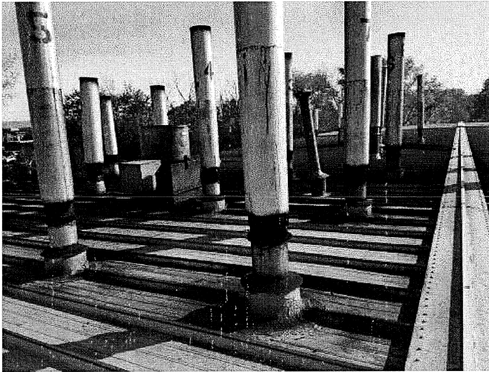
Image 20(Heat Treat Stacks) : Heat Treat Stacks with black soot on roof.
