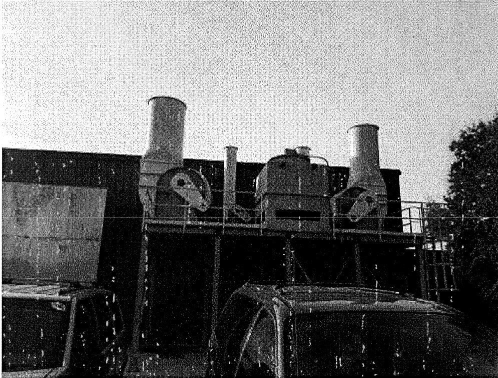
Image 7(B5 line stacks) : B5 line stacks.
