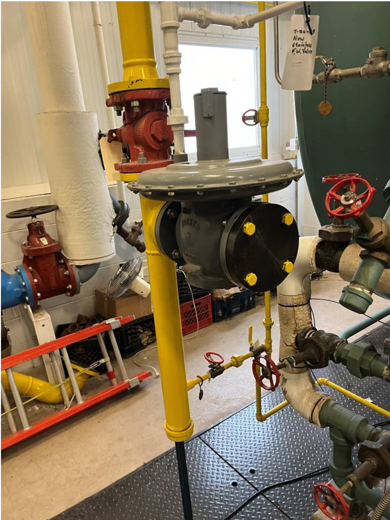
Capped natural gas fuel line to FG-BOILERS.
