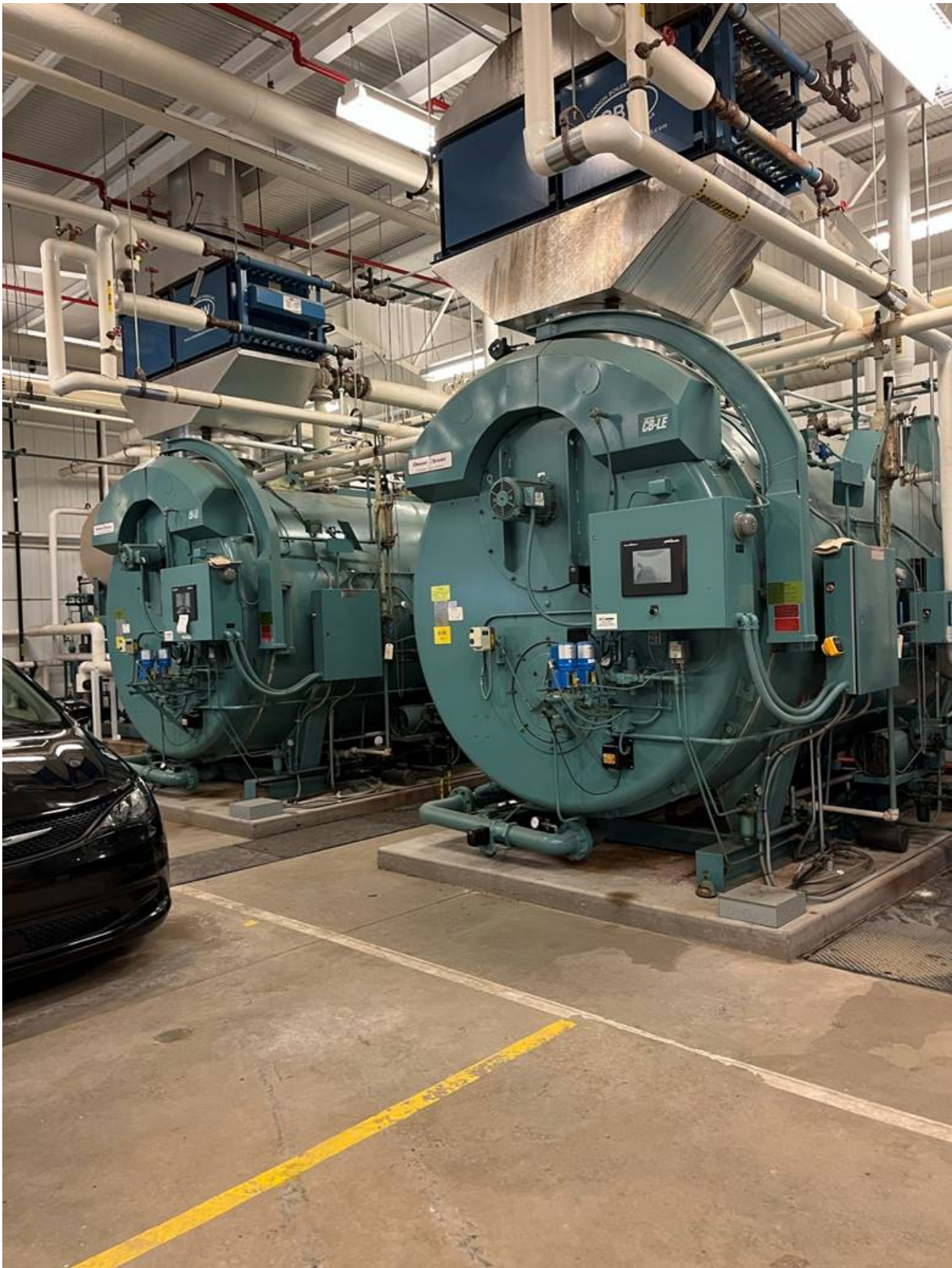
FG-BOILERS, permanently shut down.
