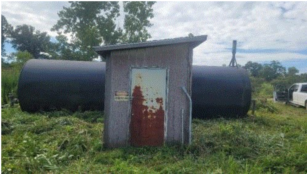
Image 2(ALF AIRSTRIPPER 1) : Verify vegetation cleared around unit
