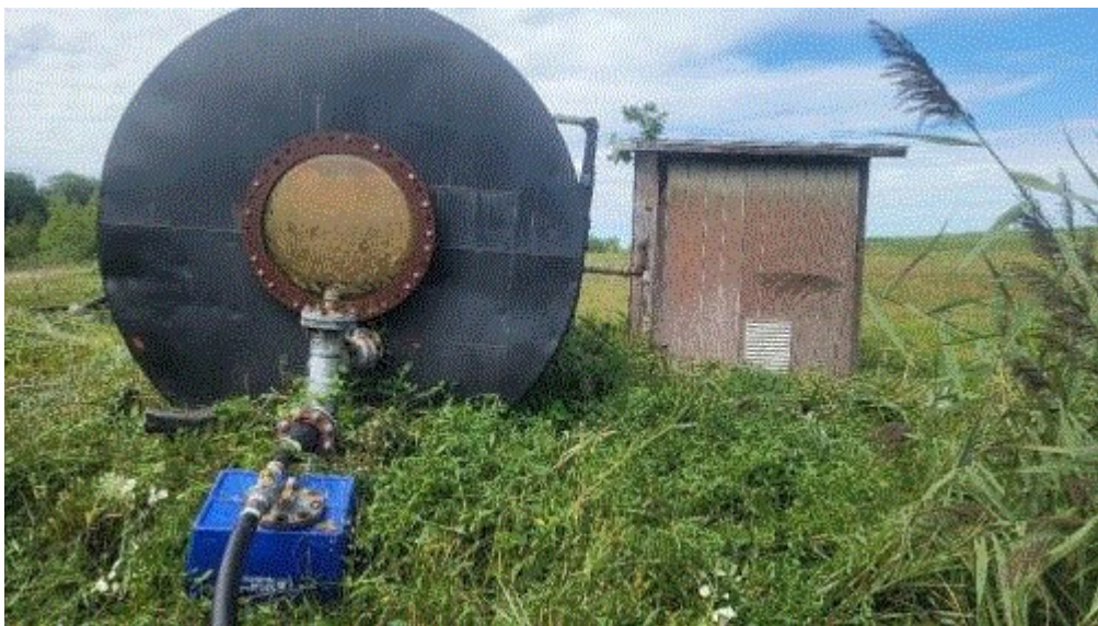
Image 3(ALF AIRSTRIPPER 2) : Verify vegetation cleared around unit
