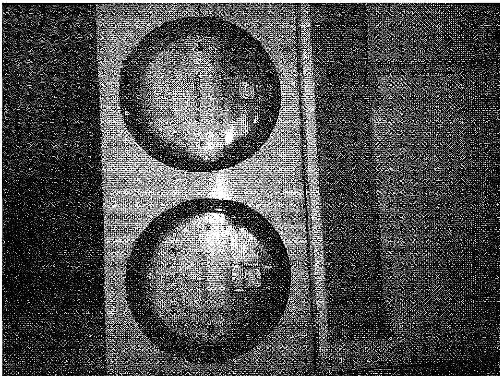
Image 5(EU-CHROMEPLATE32 Mag) : No indication of DP, scrubber and exhaust fan in-op
