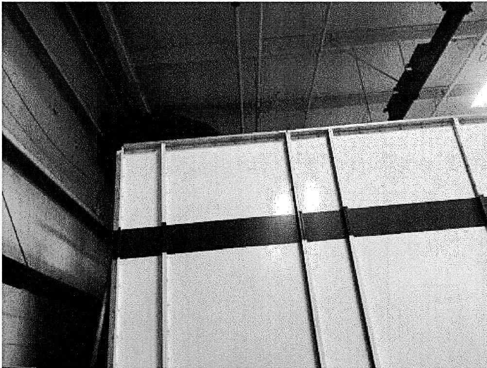
Image 3(Exhaust) : View of spray booth exhaust stack
