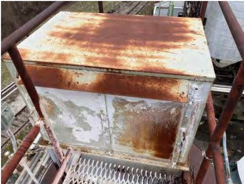
Image 1(001) : Bag filter cabinet atop lime storage silo, EULimeTank540 on 4/13/2022.
