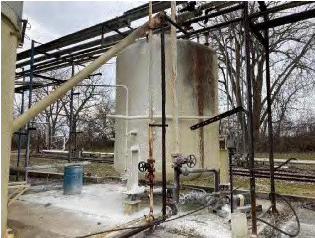
Image 2(002) : Lime slurry tank EULimeSlurry541; housekeeping issue on 4/13/2022.
