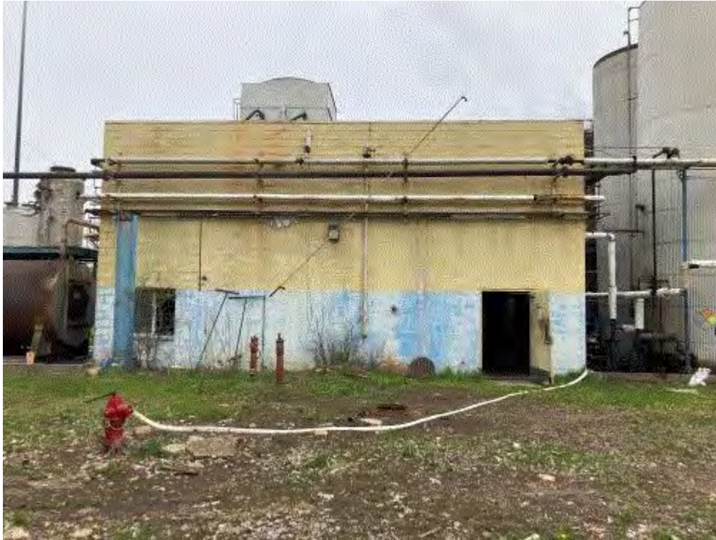
Image 4(004) : Exhaust vent for EUPilotOxidation is pipe at 45 degree angle above roofline, as seen on 5/5/2022.
