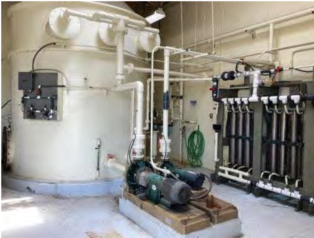
Image 2(12,000 scfm control) : Operational 12,000 scfm sodium hypochlorite odor control system with rectifier set used to convert NaCl to sodium hypochlorite
