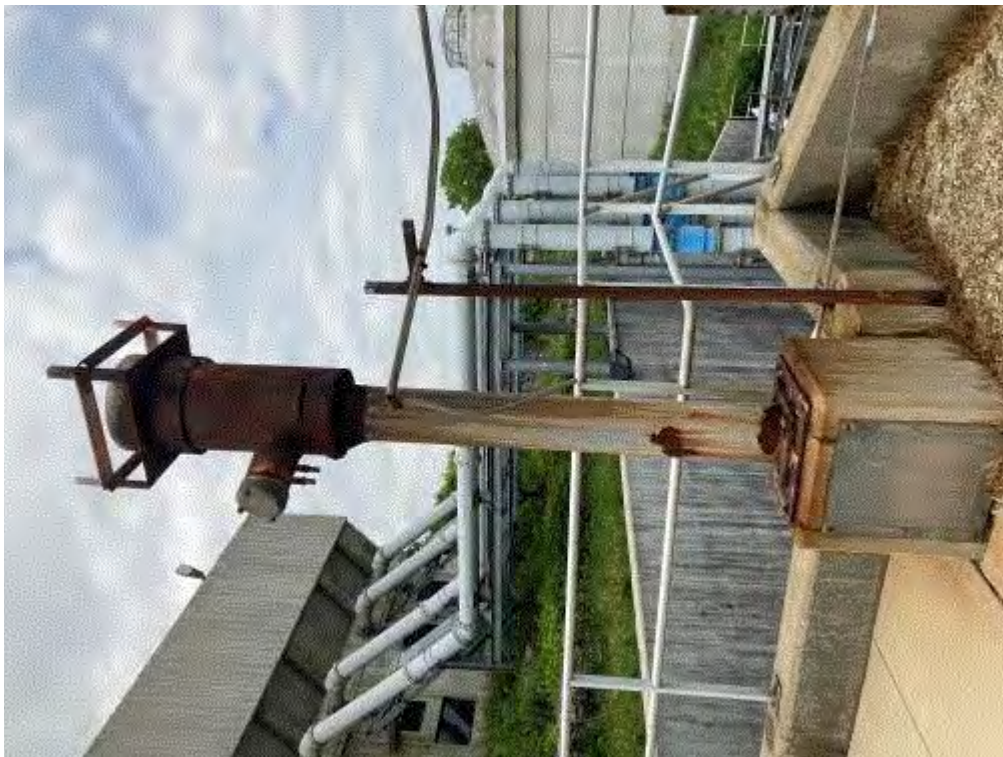
Image 3(Sour Gas Flare) : Used to combust excess digester gas
