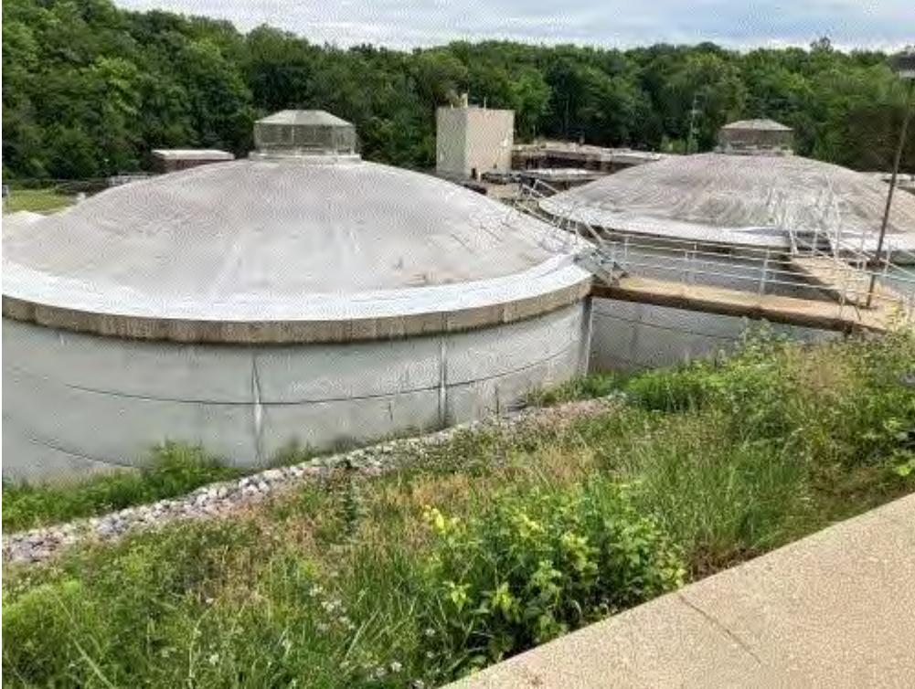
Image 4(Secondary Treatment) : Secondary treatment, covered with vents. Treated with biotowers & odors controlled with sodium hypochlorite scrubber.
