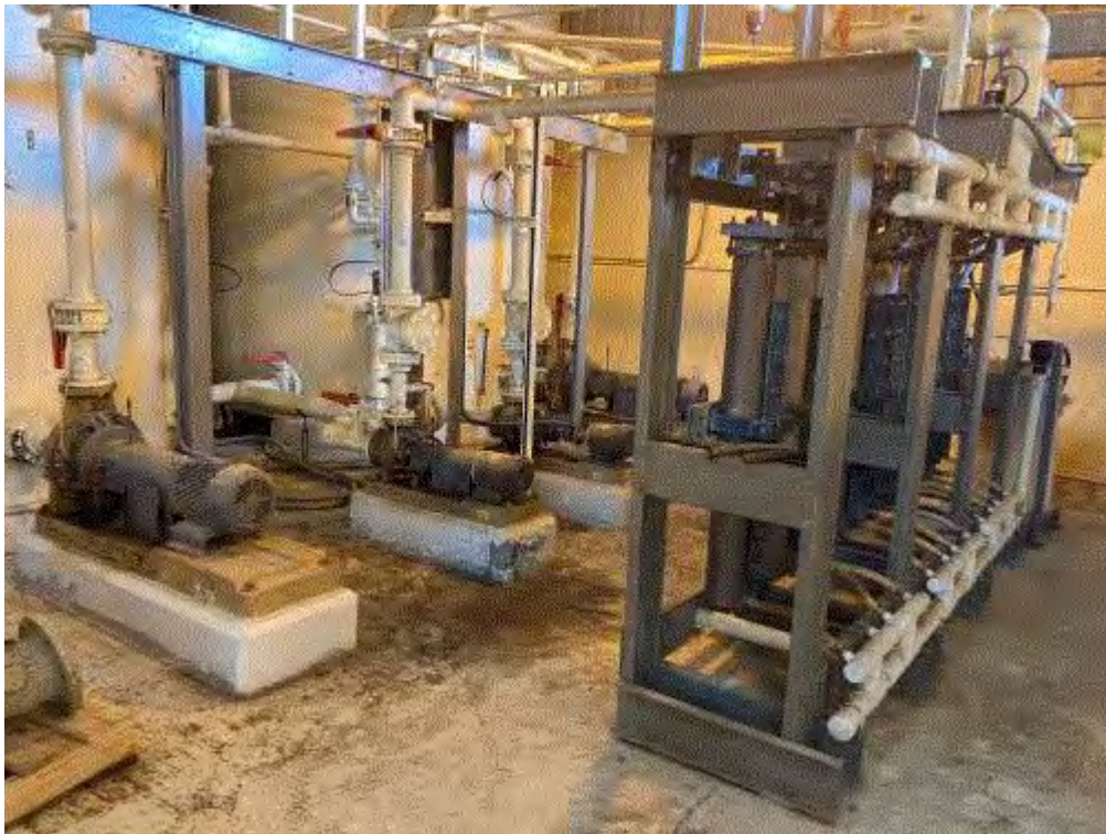
Image 1(22,000 scfm scrubber) : Two 22,000 scfm scrubbers which are no longer operational.
