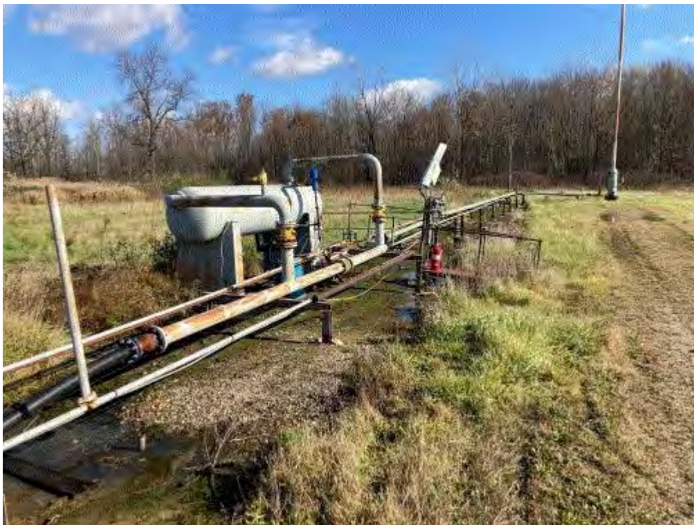
Image 2(002) : Knockout drum on way to flare.
