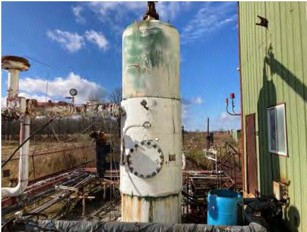
Image 1(001) : Gas plant inlet separator.
