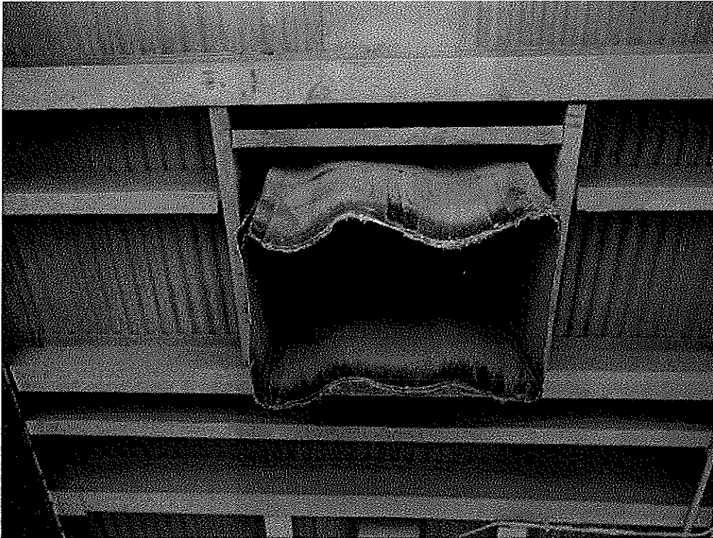
Image 9(Non-market Loadout) : Non-marketable fly ash loadout chute. Fly ash mixed with surfactant prior to loadout through chute.
