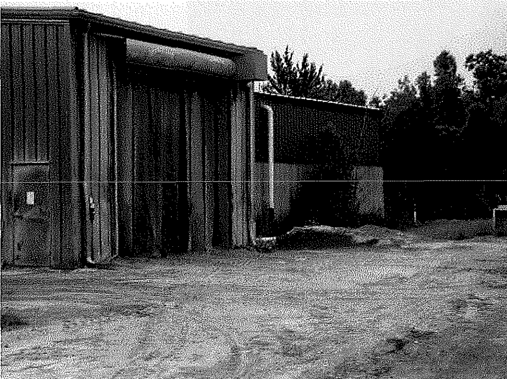
Image 3(FGASHHANDLING) : Repaired door with new seals, door rollers, new door. Front end loaders enter mass storage building through this entrance.
