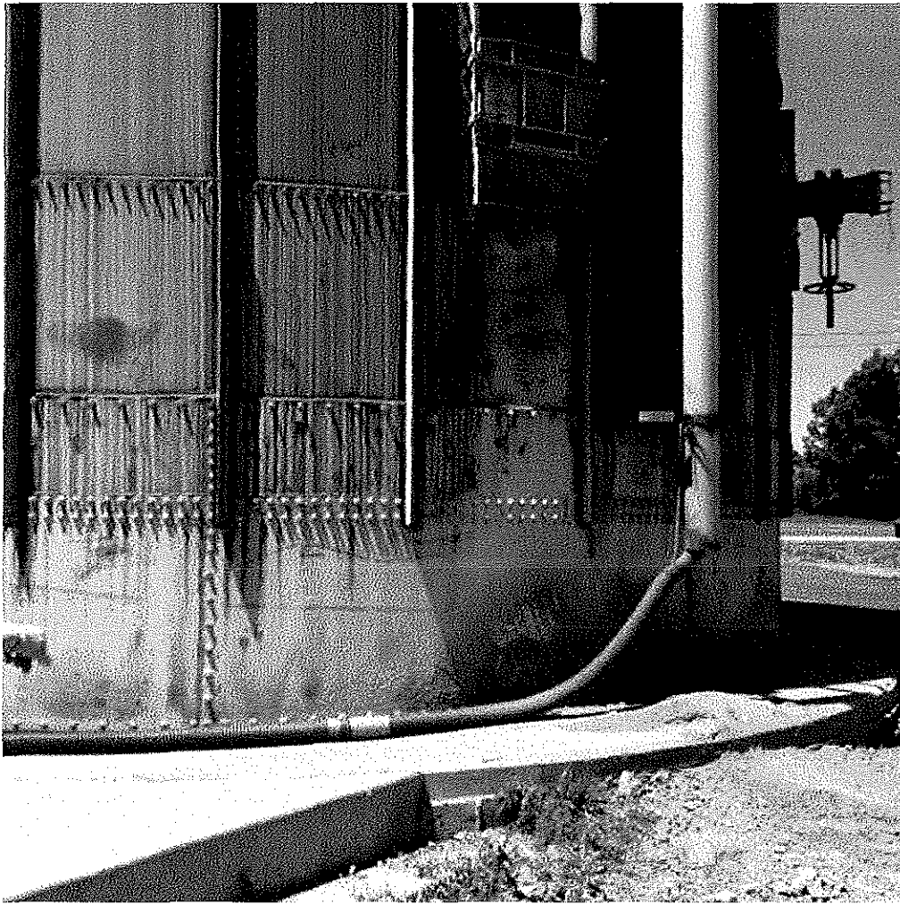
Image 5(FGASHHANDLING) : Storage silo with ventilation piping. Appears to be "leaking" fly ash onto cement pad.
