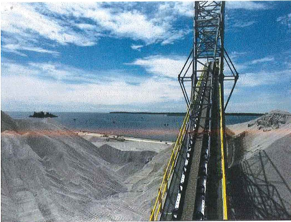
Image 3(Belt Conveyor) : New belt conveyor
