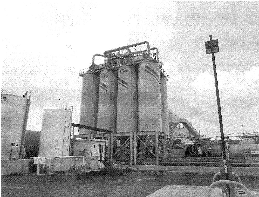
Image 1(P1240267.JPG) : View of HMA silos from the north with top mounted fugitive emission capture system that was installed on top of the silos between the 2012 and 2013 production seasons.
