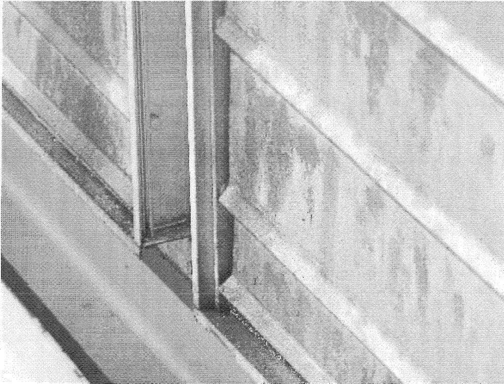
Image 6(P1240292.JPG) : Close-up view of post particulate control condensation on the exhaust louvers. Control system is undergoing engineering review to correct this issue.
