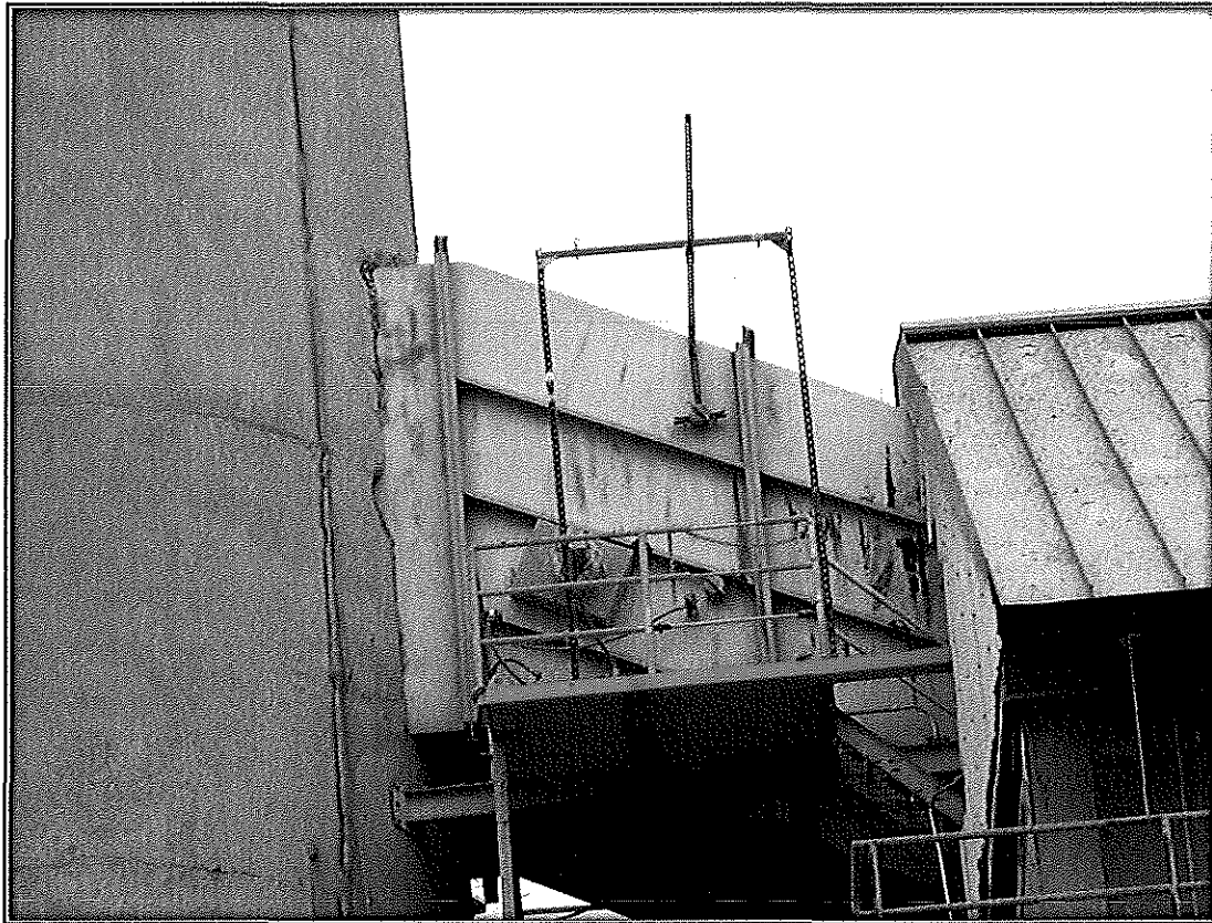
Figure 4-2. Kiln 19 Breaching Duct
