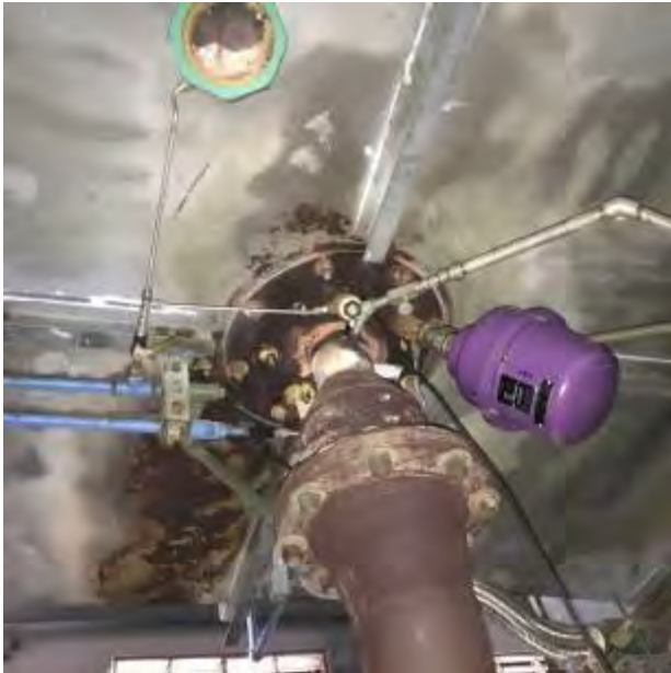
Burner area is hotter than normal need to monitor
