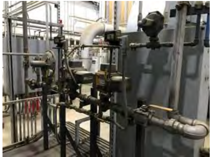
No gas smell around the burner gas train
