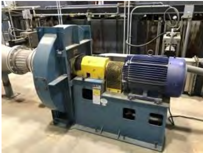
The RTO supply fan operate normal no issues observed
