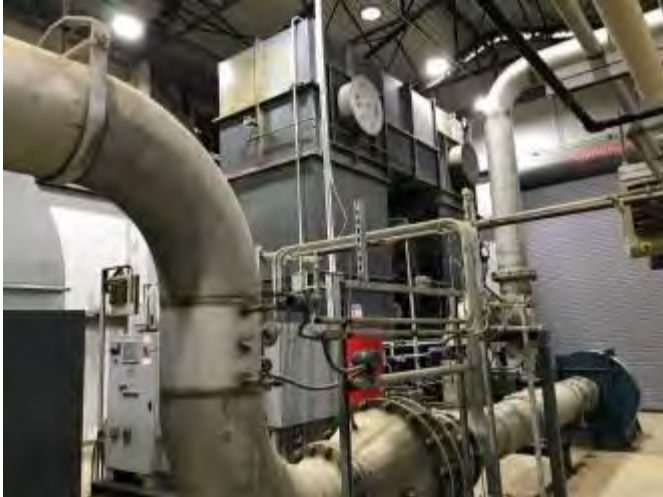
The Met Pro 2 Tower RTO at Aria Energy
