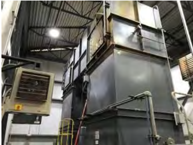
Hot spot observed on outlet side of the RTO system
