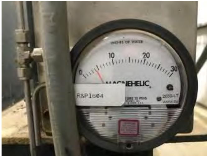
RTO differential pressure gauge 4.25" during online inspection no indication of excessive plugging at this time
