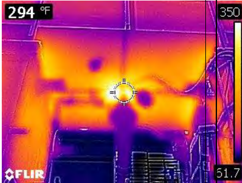
Infrared photo of burner area online
