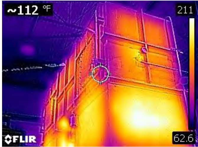
Infrared photo of outlet side RTO online no major hot spots
