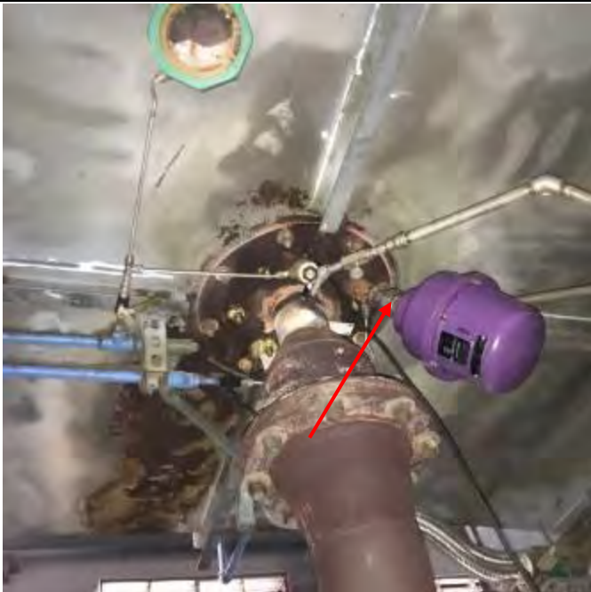
Build-up on burner site glass indicates particulate build-up is happening on UV scanner needs to be cleaned often to stop burner flame fault issues.
