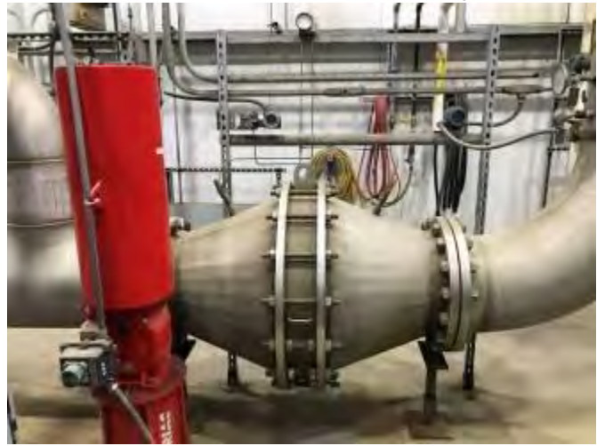
Flame arrester must be clean very little differential pressure drop
