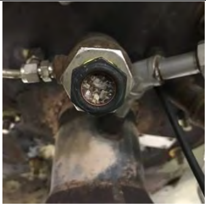
Close up of burner site glass.
