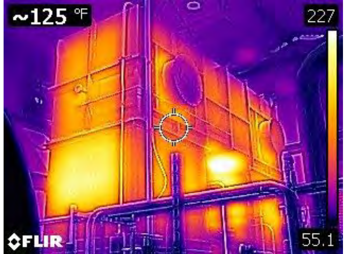
Infrared photo of inlet side RTO online no major hot spots
