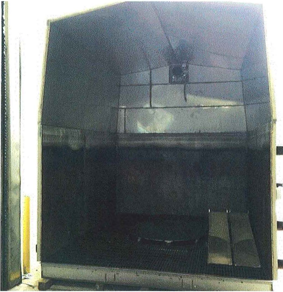
Image 3(Cleaning Booth) : Internal view of cleaning booth that is vented to outside ambient air
