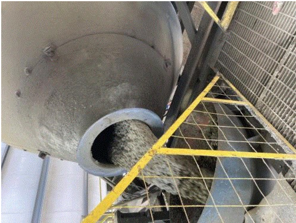
Image 6(Picture 6) : Unloading Concrete from the central mixer and loading to truck drum
