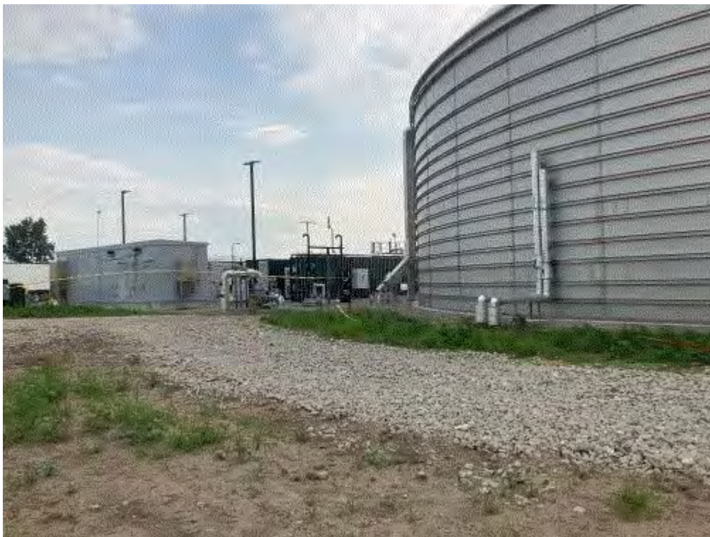
Image 4(Site) : Photo of anaerobic digester (right) and EUGCU (left & center).
