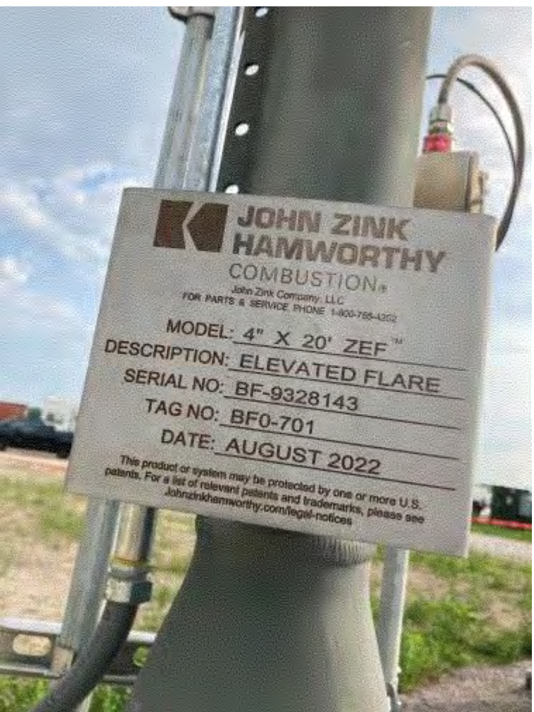
Image 2(Flare Nameplate) : John Zink biogas flare nameplate
