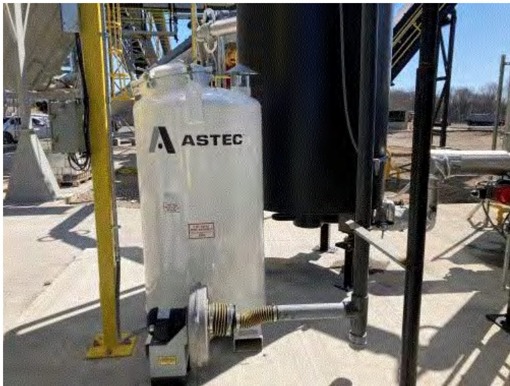
Image 1(001) : Astec condenser control device shared by 6 liquid AC storage tanks.
