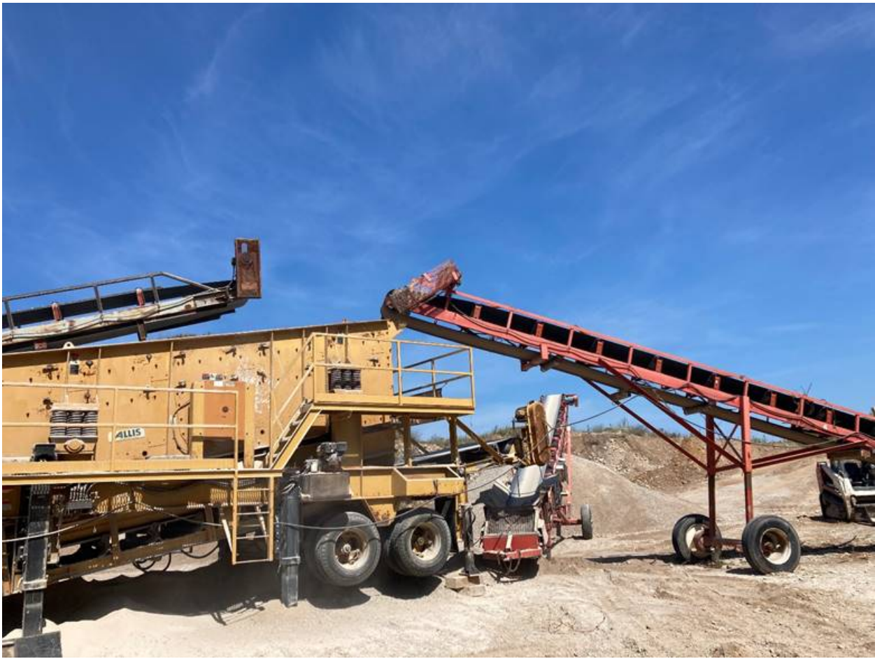
Image 1: Allis screen and conveyors
