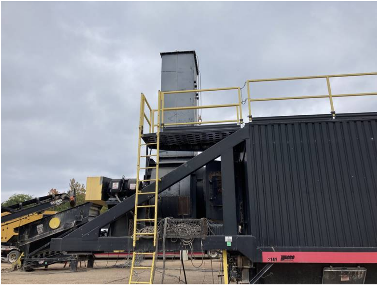
Image 2: Baghouse and stack
