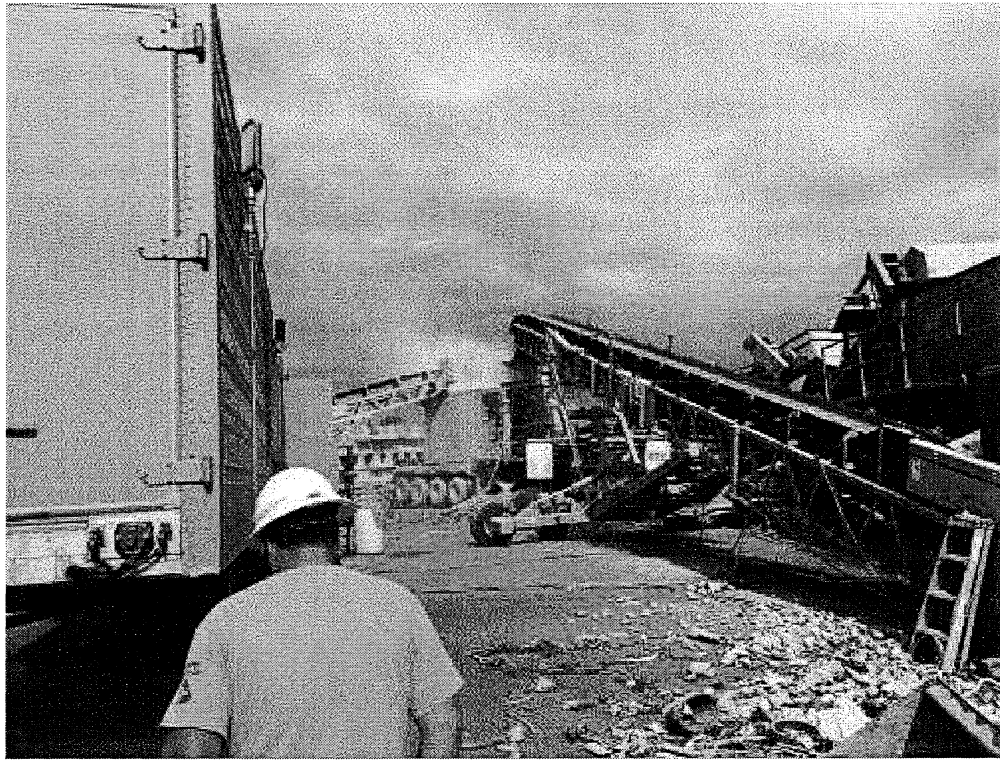
Image 1(KPI 4250) : Walking up to the job site. Excessive VEs observed.
