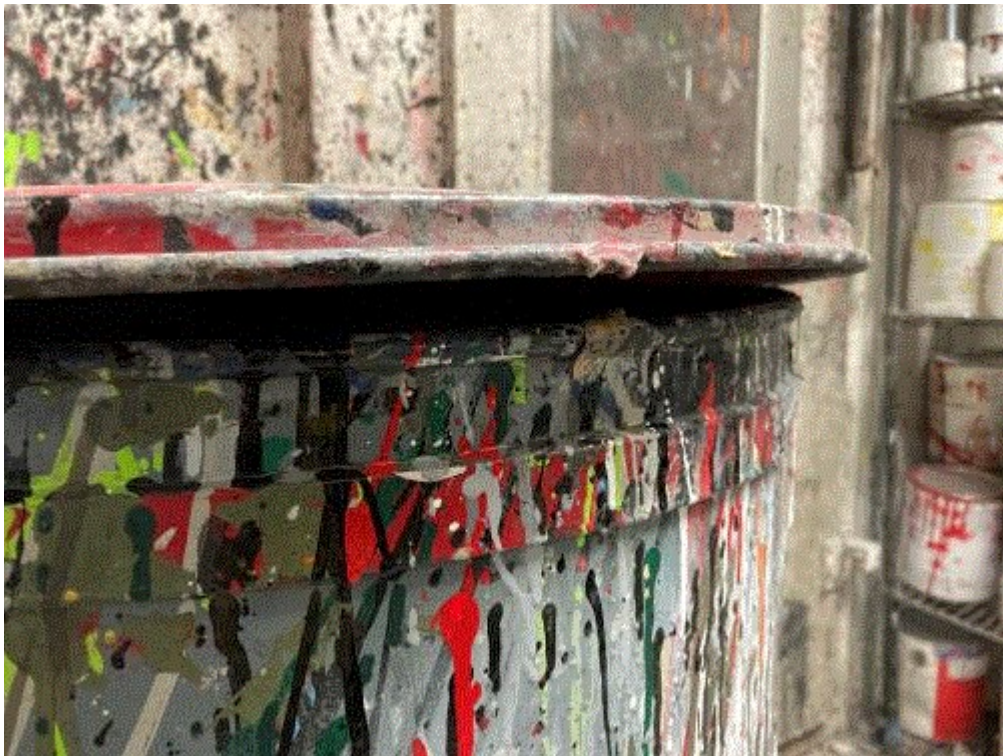
Image 11(IMG 0436) : Close-up view of drum lid in the full closed position. Note that the lid does not rest flush against the lip of the drum. This waste drum appeared to be the source of fugitive emissions, which caused a strong solvent odor in the paint room.
