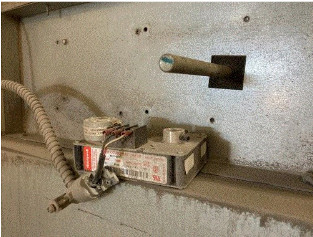
Image 6(IMG_0421) : EUBOOTH2. Close-up view of the west booth air balance actuator, which was removed from the damper control rod.
