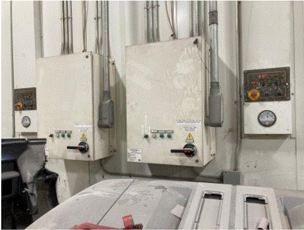
Image 7(IMG 0431) : EUBOOTH2 west (left) and east (right) control panels, each with a circular booth air balance gauge.
