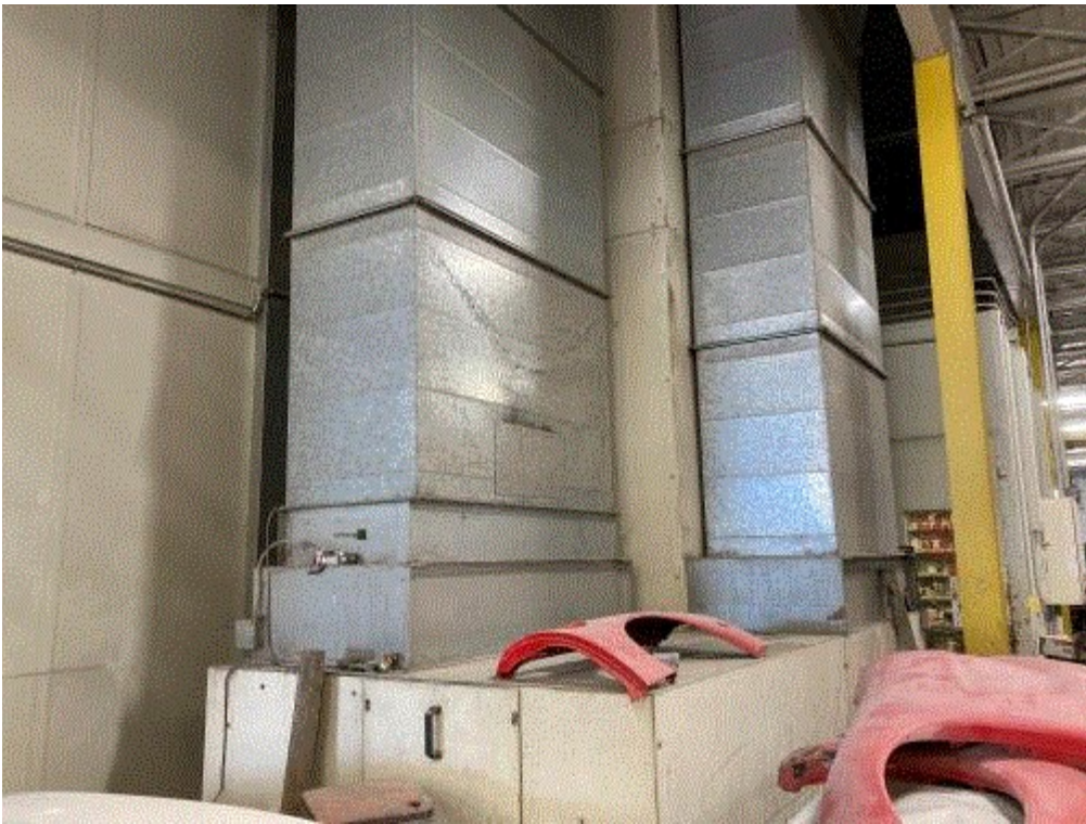
Image 5(IMG_0420) : EUBOOTH2 west booth ductwork. The west booth air balance actuator is disconnected from the damper. IMG_0421 provides a close-up view.
