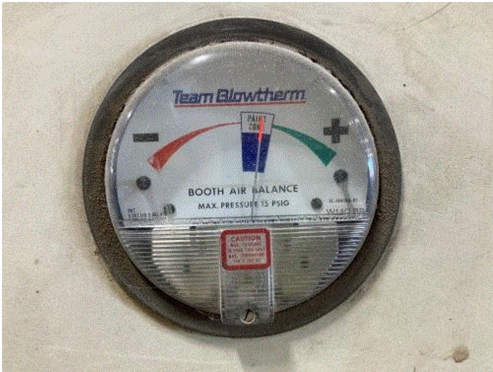
Image 3(IMG 0417) : EUBOOTH1 booth air balance gauge. The orange-tipped indicator needle moves to the right side of the "Paint Zone" when the exhaust is turned on. This appears to indicate the pressure differential is within the manufacturer's specifications.
