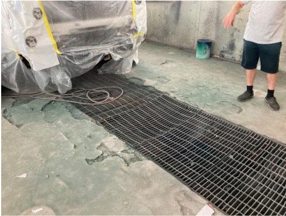
Image 12(IMG 0441): EUBOOTH2. View of the downdraft exhaust floor grates. The floor grates have been cleaned of material that obstructed the exhaust. All of the PM exhaust filters in EUBOOTH2 appeared to be properly installed.
