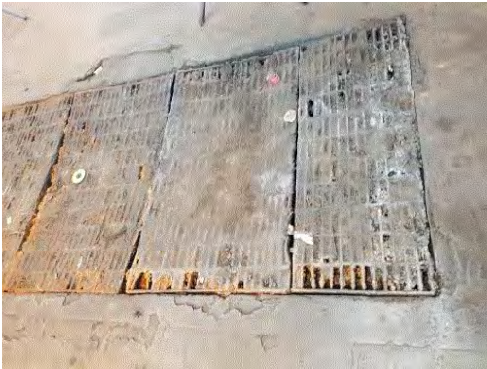
Image 1(GRATE 1 OF 2 2020080) : Section of floor grate covering dry particulate exhaust filter. Note that air flow through the grate is mostly obstructed.
