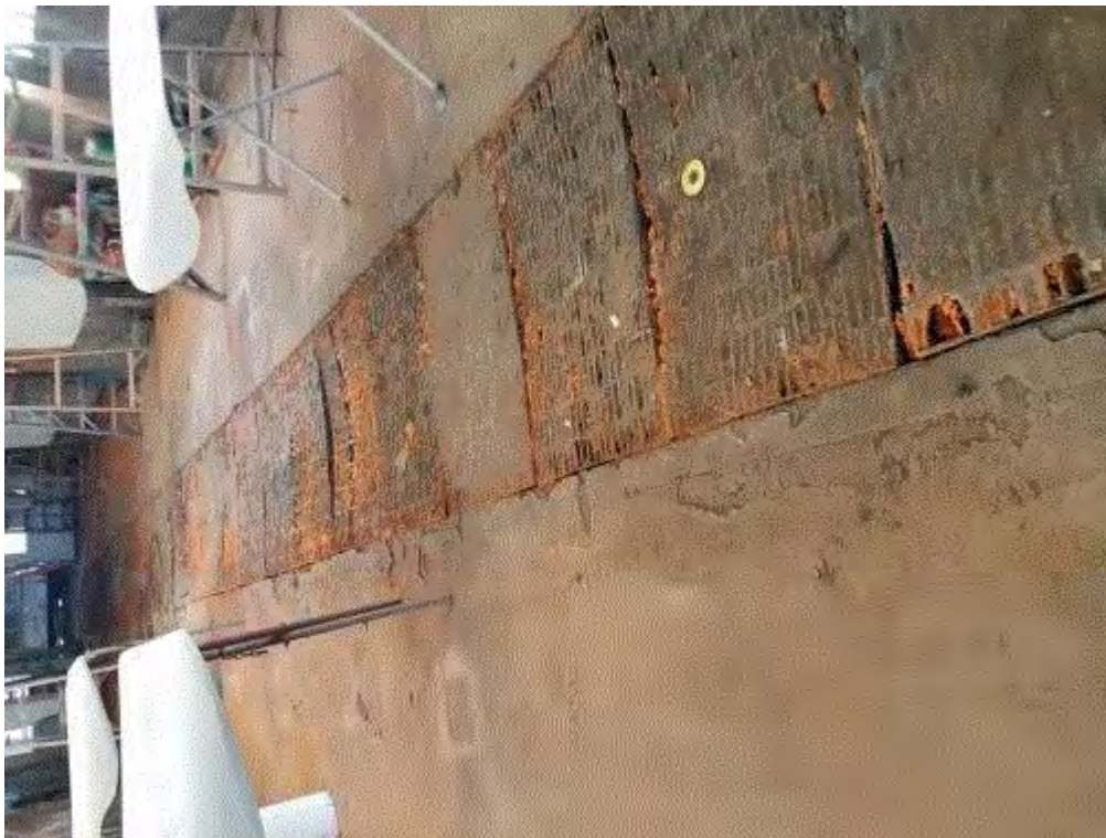
Image 2(GRATE 2 OF 2, 202008) : Floor grate covering dry particulate exhaust filter. Note that air flow through the grate is mostly obstructed.
