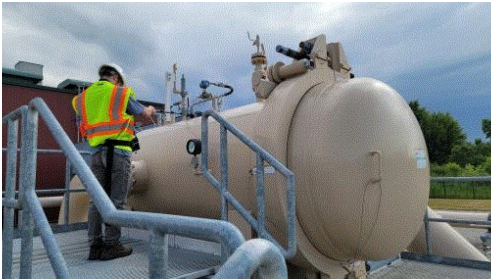
Image 2(Leak Location) : Leak location on top of tank.
