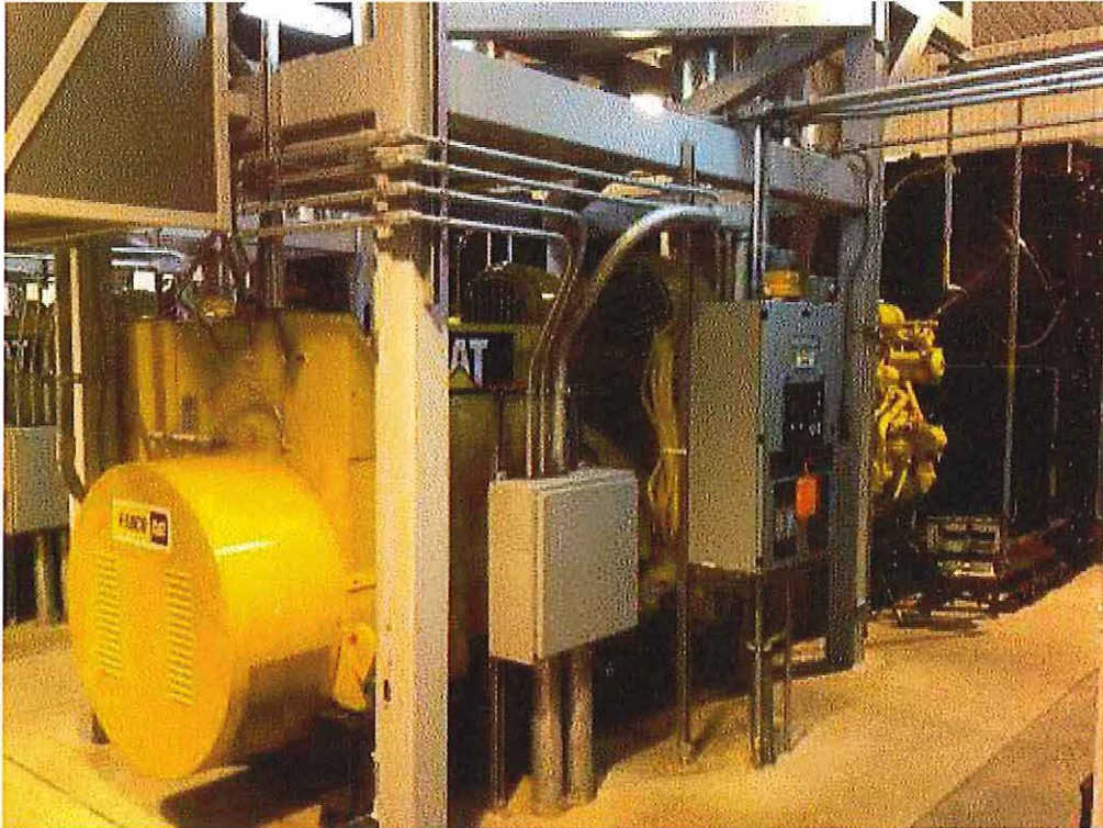
Image 7(MTU7) : Cat diesel/biodiesel generator set
