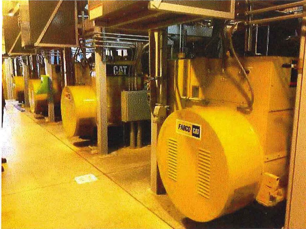
Image 5(MTU5) : Cat diesel/biodiesel generator units
