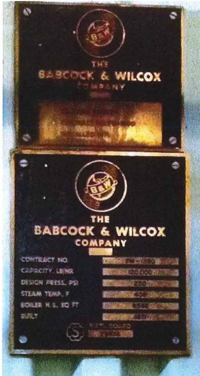
Image 4(MTU4) : Boiler ID Plates
