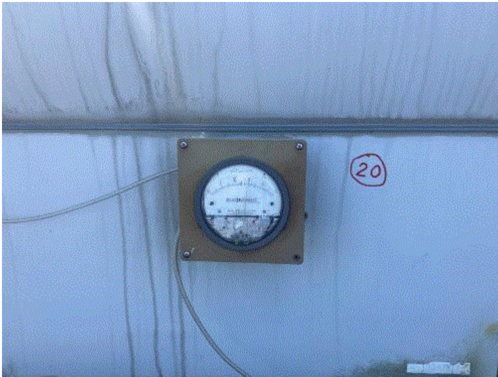
Image 6(Nitric Line) : Nitric Line pressure drop gauge.
