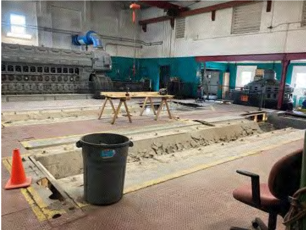
Image 1(Engines Removed) : Areas where EUENGINE2 and EUENGINE3 have been removed from facility
