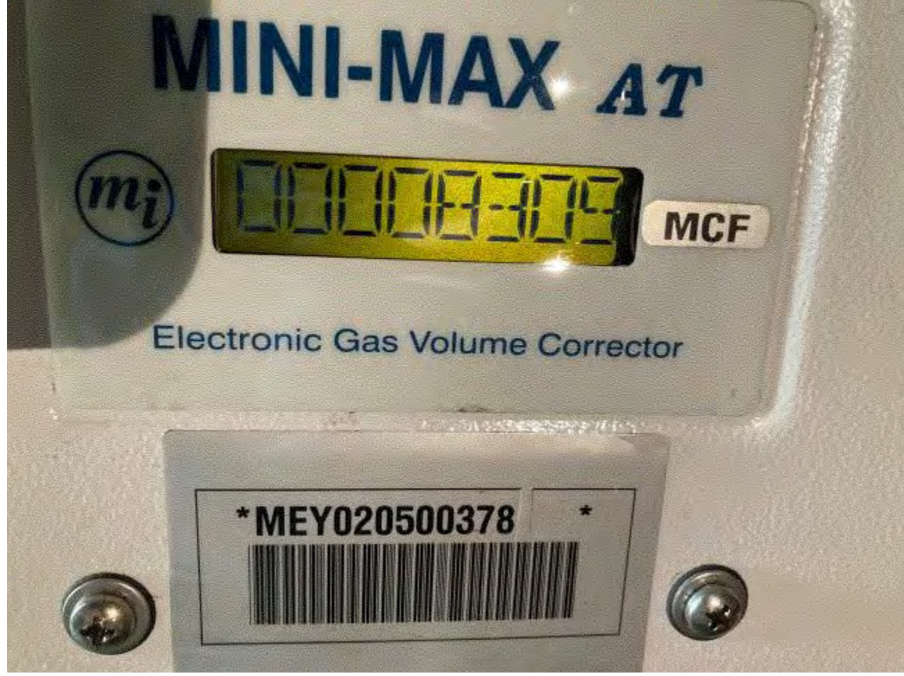
Image 7(Natural Gas) : Natural Gas Meter for EUENGINE1 & EUENGINE7
