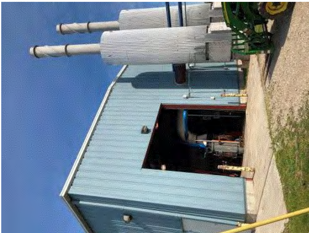
Image 9(FGENGINE89) : Building housing EUENGINE8 and EUENGINE9
