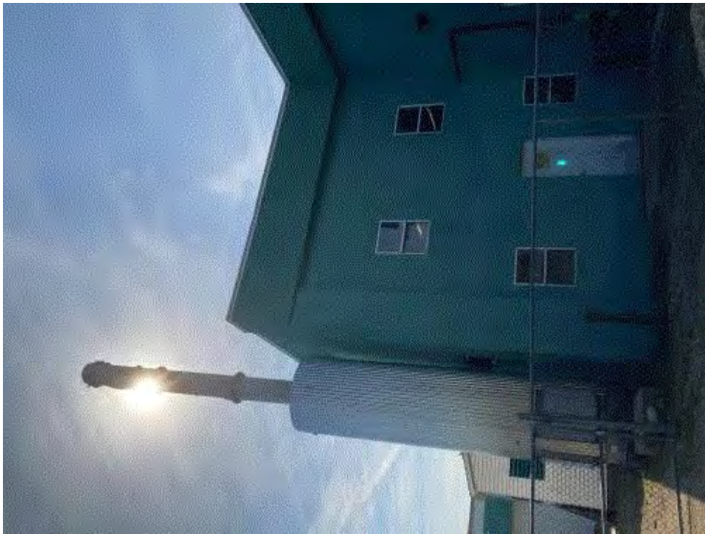
Image 8(EUENGINE7 Stack) : Stack on EUENGINE7
