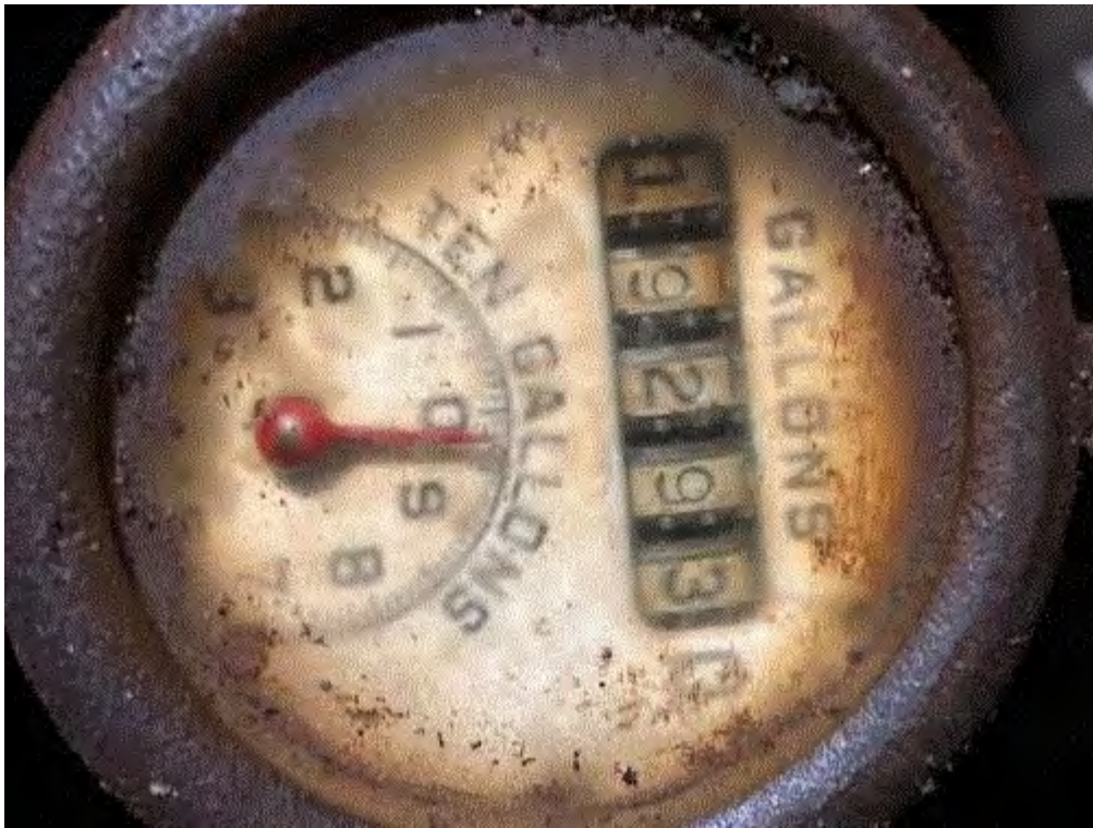
Image 2(Diesel #1) : Diesel Monitor on EUENGINE1
