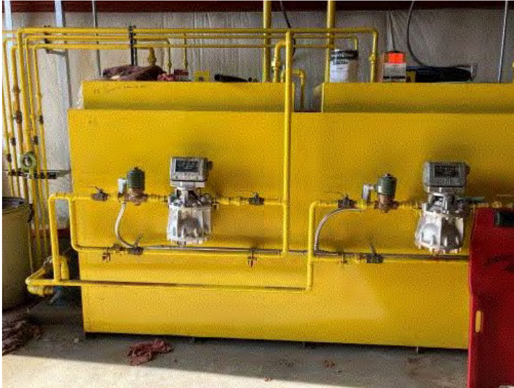
Image 4(Diesel 8&9) : Diesel Tanks for EUENGINE8 & EUENGINE9
