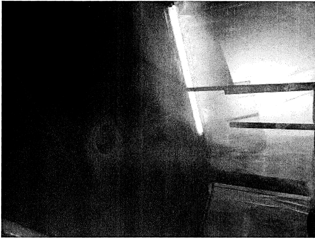
Image 10(Hot Wire Exhaust) : Photo of exhaust inside hot wire cutting booth; Provided by Lisa Bascom of Brooklyn Products
