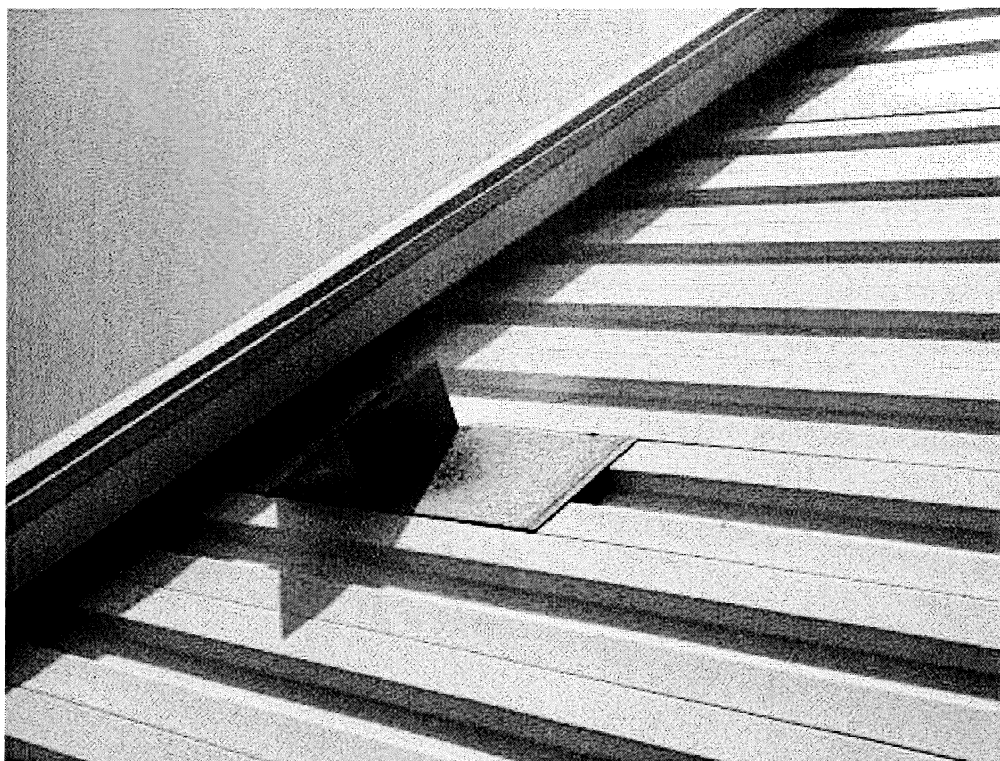
Image 12(Hot Wire Exhaust) : Exterior exhaust while hot wire cutting booth was in operation; Photo provided by Lisa Bascom of Brooklyn Products.
