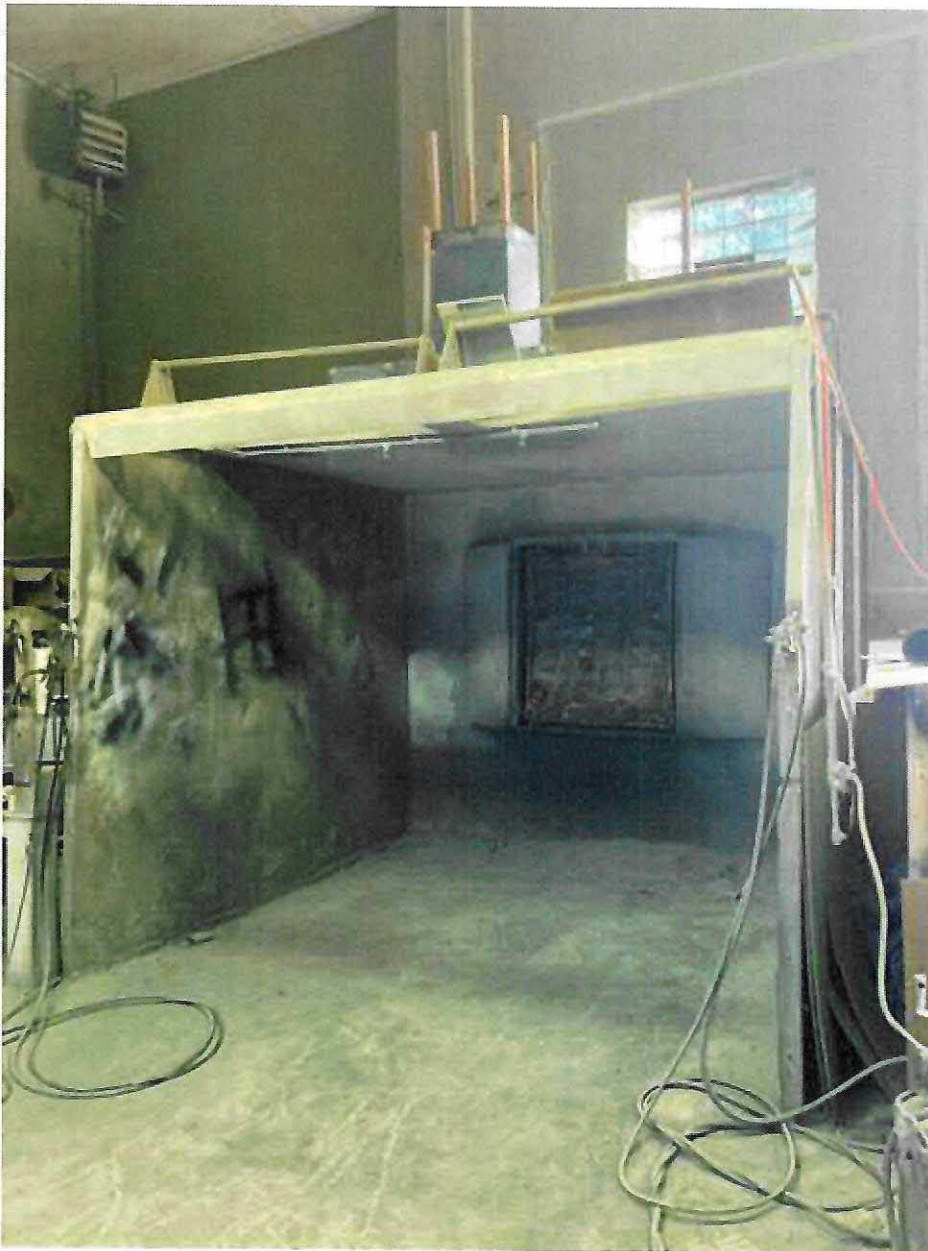
Photo Description: Spray Booth
