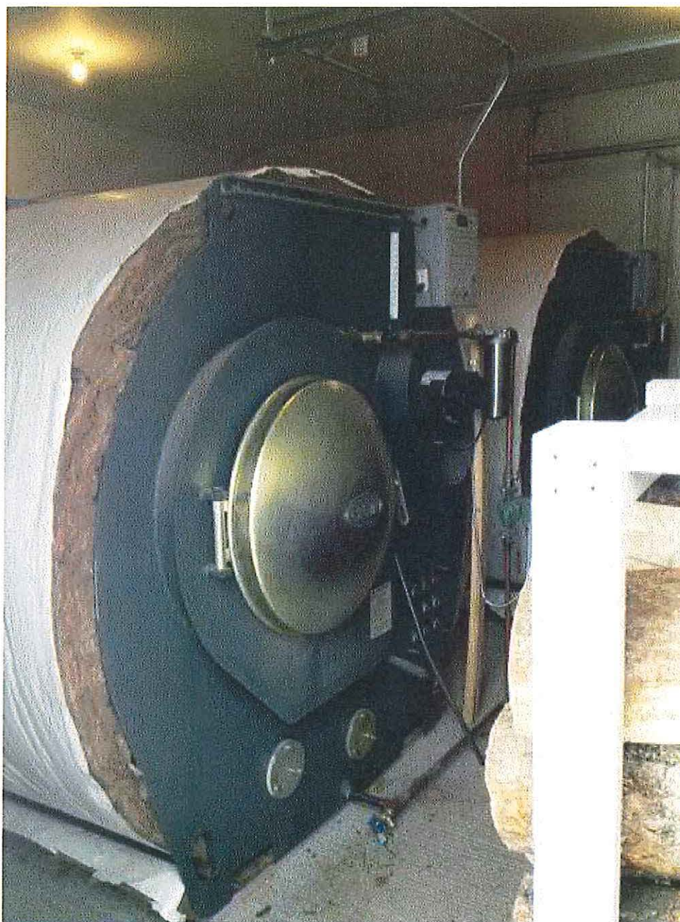
Image 7(CF5) : Two Garn wood-fueled hydronic heaters
