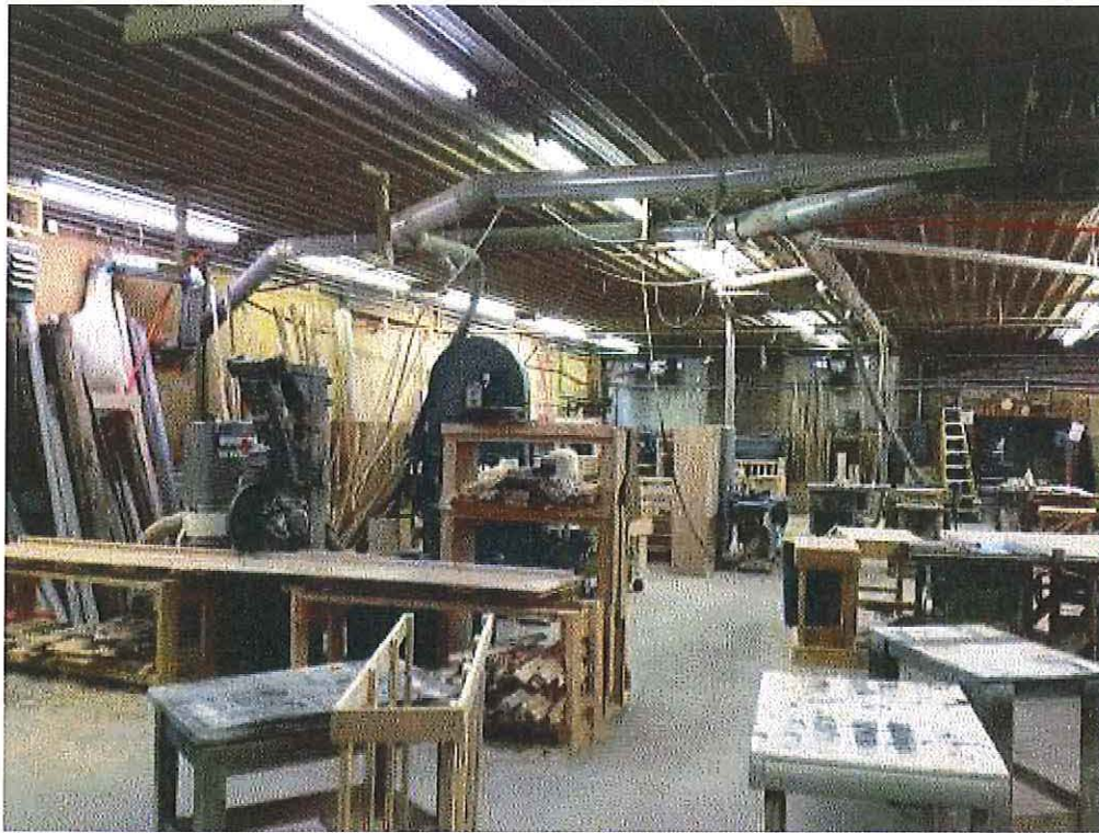
Image 4(CF2) : Wood waste collection system
