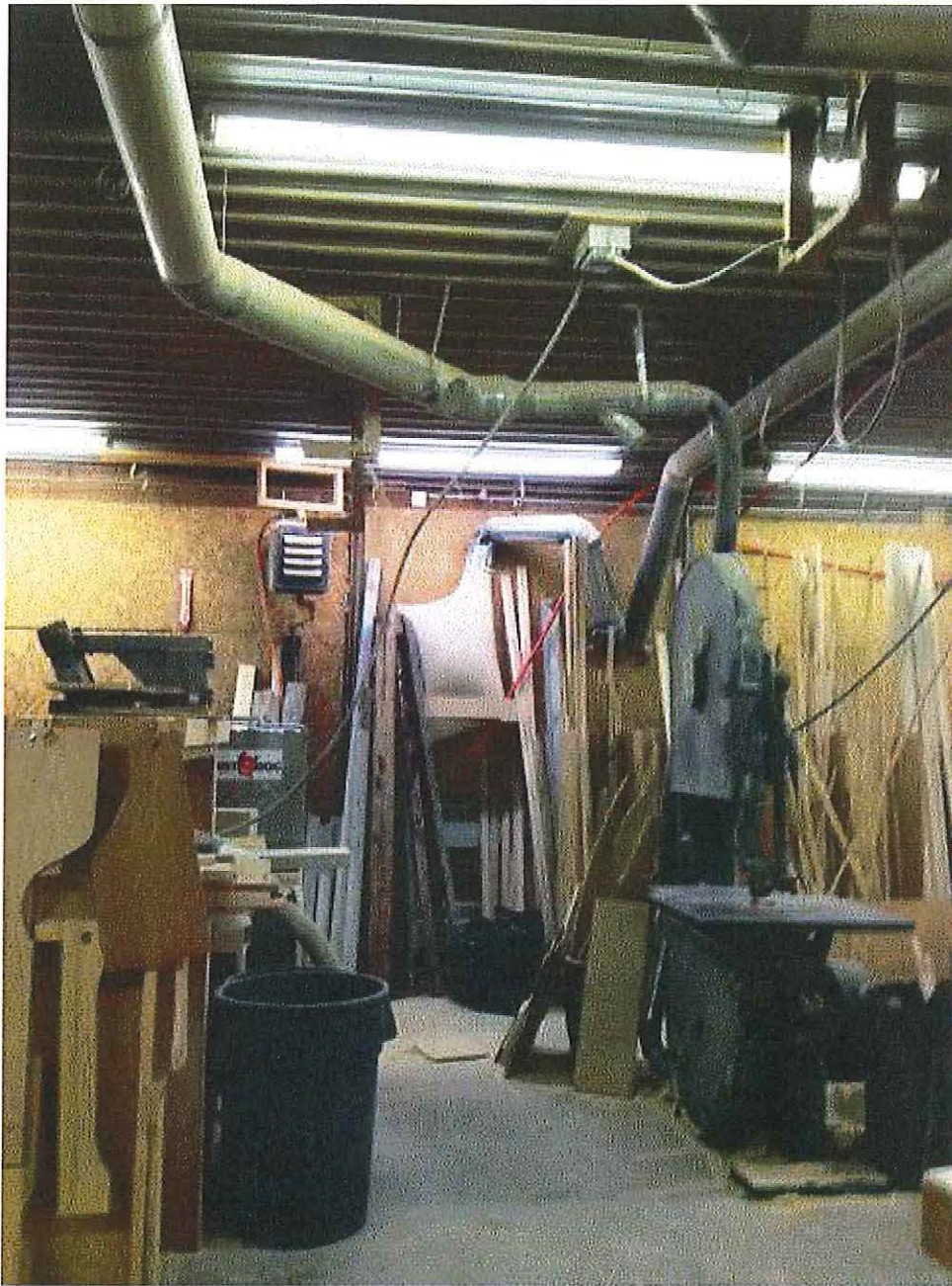
Image 3(CF1) : Wood waste collection system
