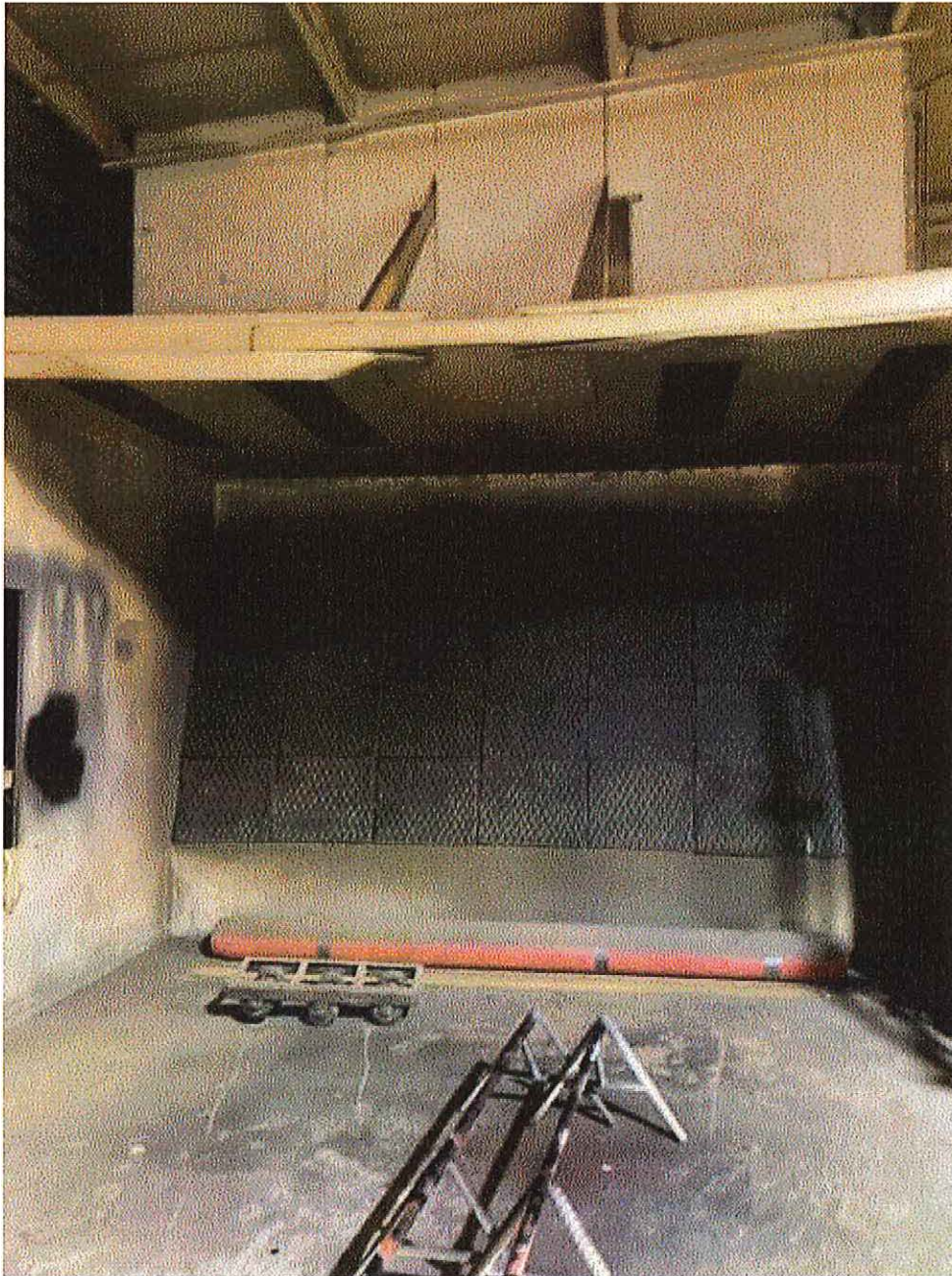
Image 2(Spray Booth) : Filters inside the spray booth
