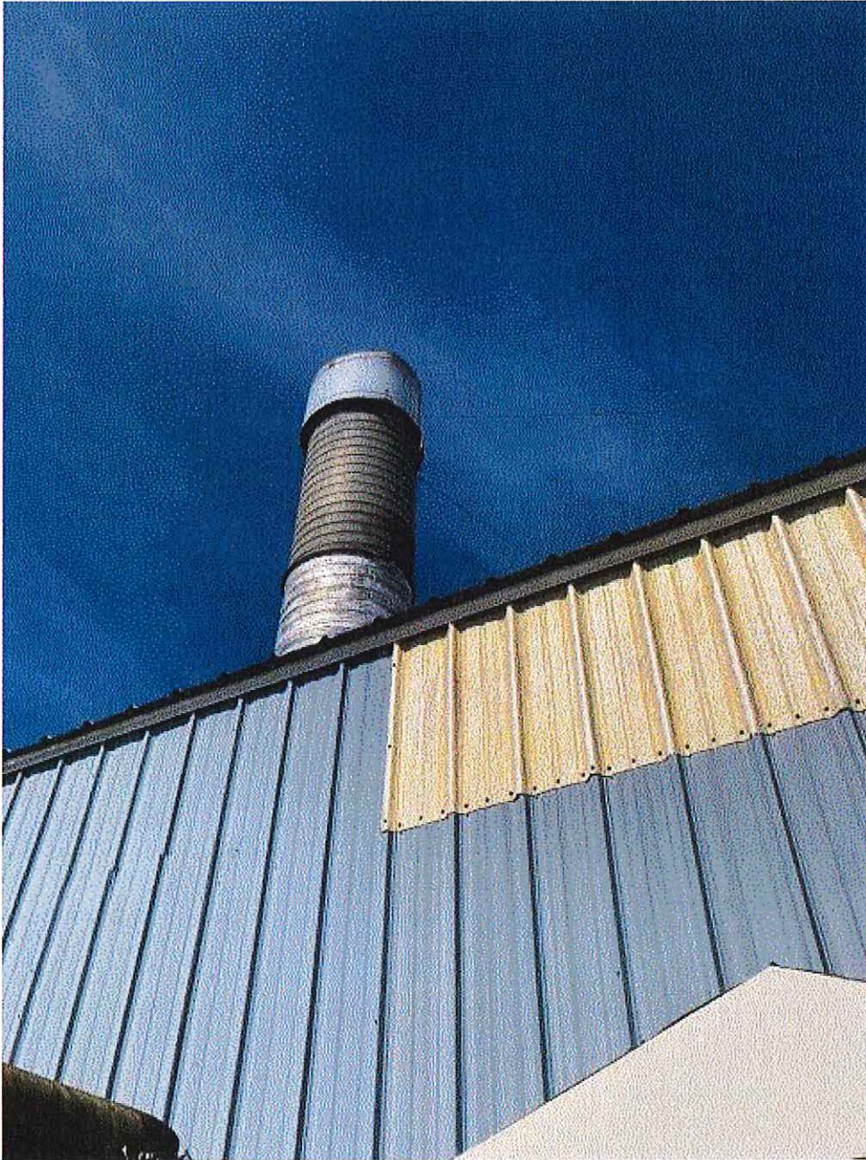
Image 1(Paint Booth Stack) : Stack from Paint Booth
