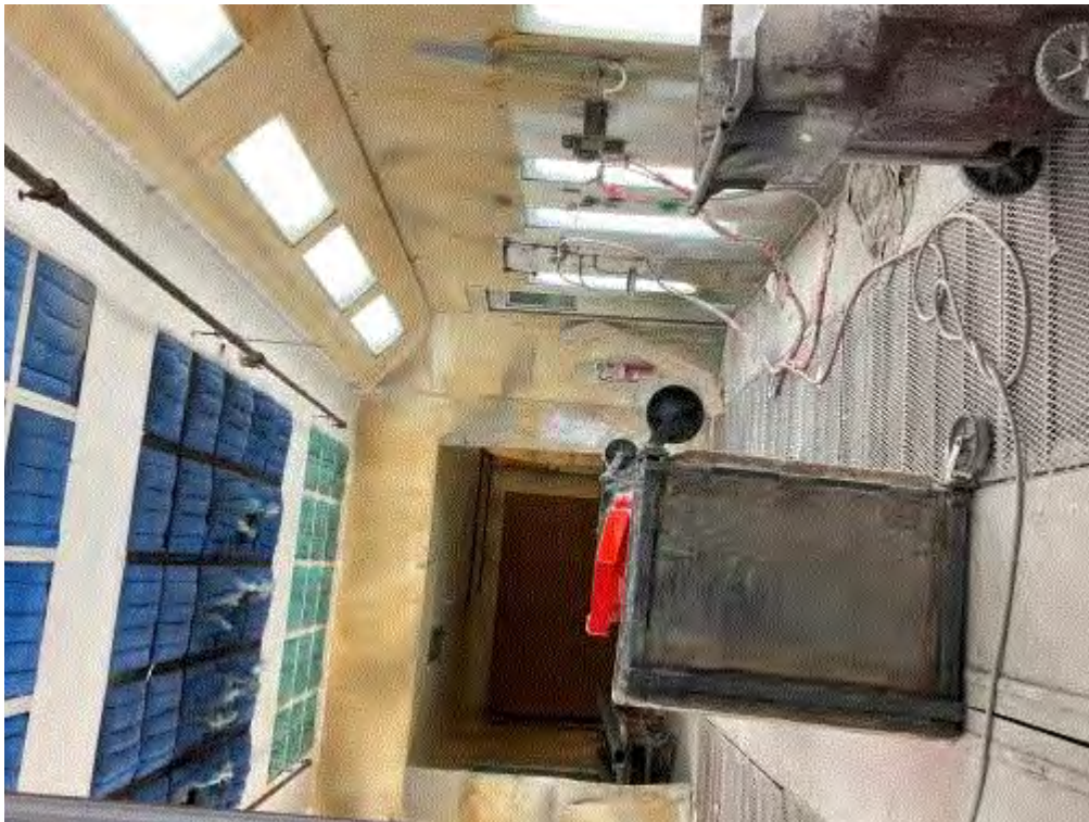
Image 12(EUEXTRABOOTH) : EUEXTRABOOTH with exhaust filters under floor panels.
