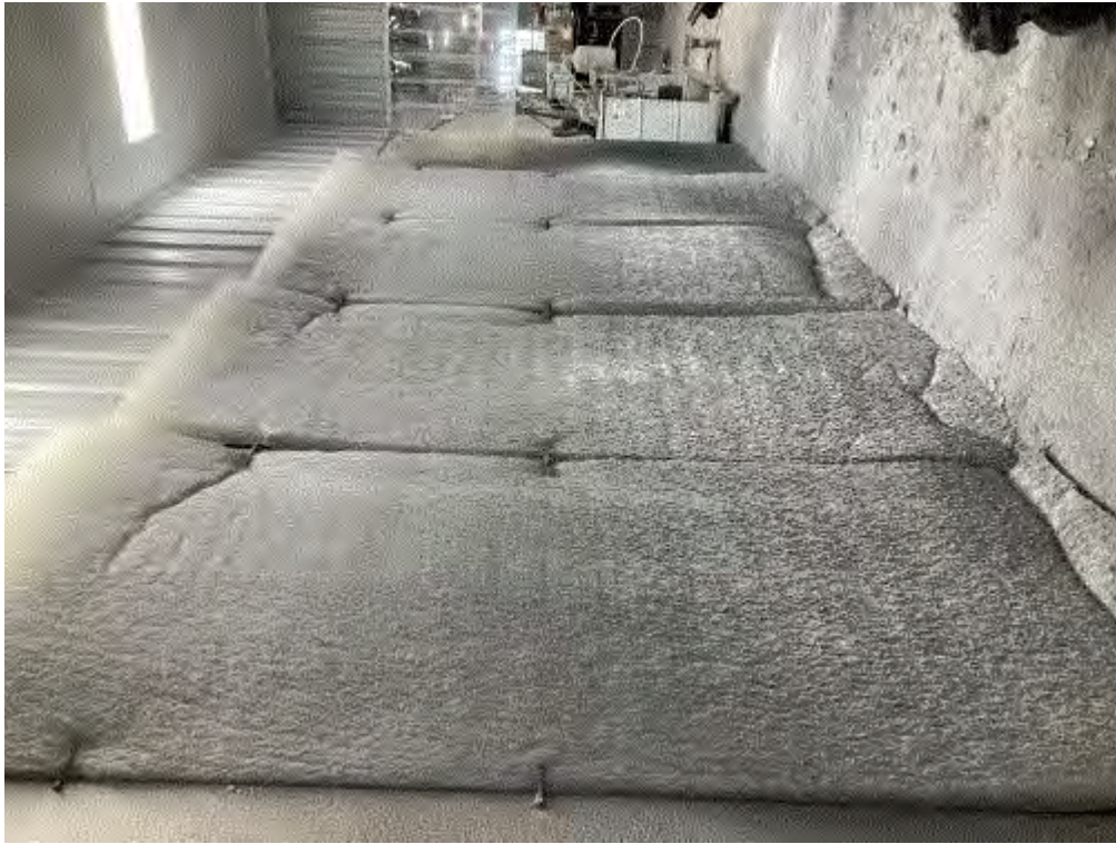
Image 8(Gelcoat Filters) : Filters installed in a gelcoat booth
