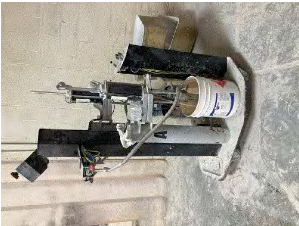
Image 5(EUADHESIVEDISPING) : EUADHESIVEDISPING emission unit. closed-loop system.
