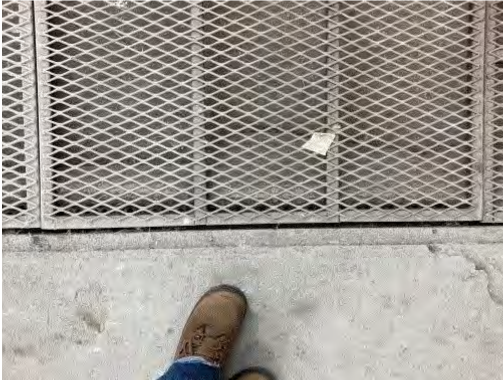
Image 13(EUEXTRABOOTH panel) : Gaps between exhaust outlet and filter media. No coating operations conducted at the time.
