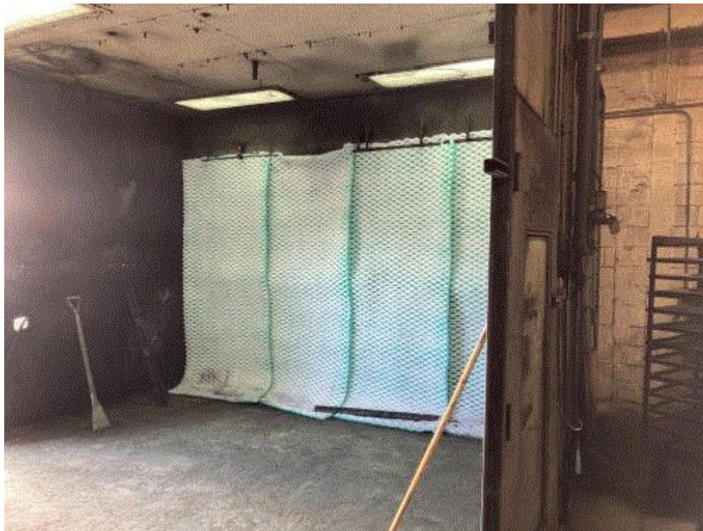
Image 1(EUBATCH2 Spray Booth) : Photo of EUBATCH2 dry filter particulate material control device. Gaps in filter placement resulted in gaps that allow particulate material to bypass the control device.
