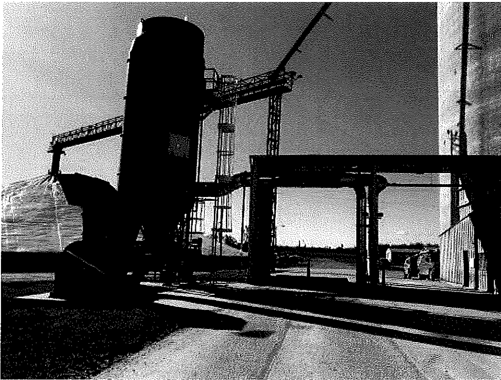
Image 1(0162) : Grain receiving Pits 1 & 2 with baghouse
