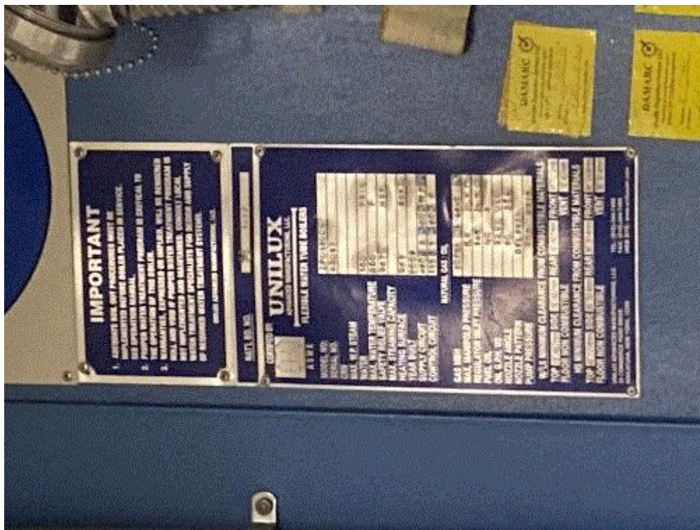
Image 7(Boiler 3) : Serial number and rating
