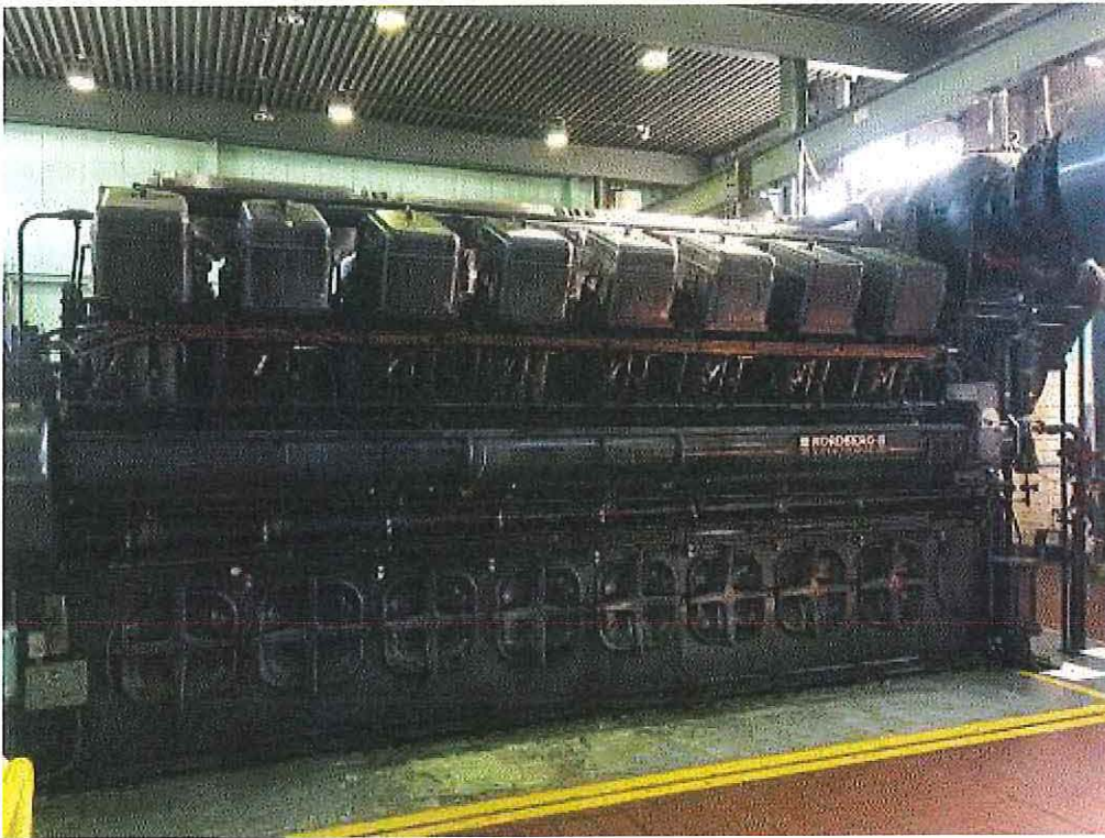
Image 2(EUENGINE4) : Nordberg FS-1316-HSC diesel generator.
