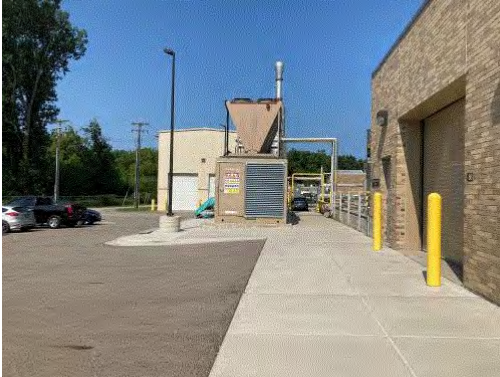
Image 4(CHP Engine) : Photo credit: Erica Shuff. Structure in middle of photo is the CHP engine.
