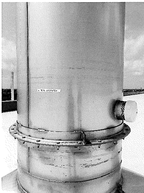
Figure 3.1.1.1: Primer Observation Zone Exhaust
